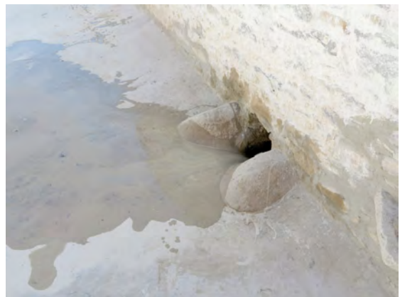
Fig. 29.3 Lhasa. Gyüme Dratsang. A water proof sprout after finishing the upper surface.
