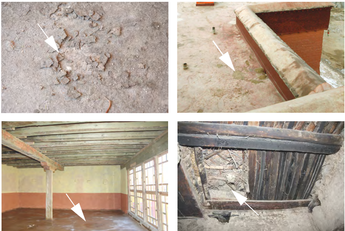
Fig. 45.3 (Top, left) Basgo. Ladakh. Serzang Lhakhang and Fig. 46.3 (Top, right) Khorchag. Ngari. Lhakhang Chenmo. Damage: Both examples showing a detaching of the upper layer of the arga surface.
