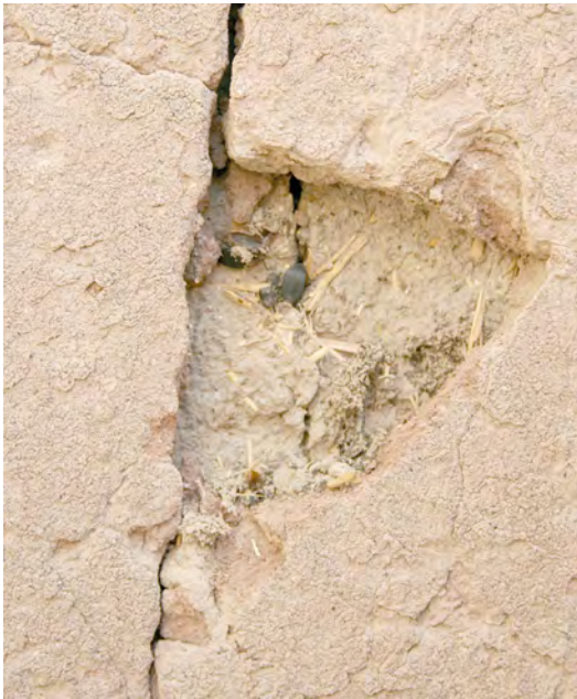
Fig. 32.2 Ne. Ladakh. Wall of a temple with missing roof. Nest of insects.
