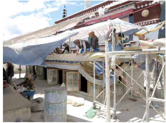
Fig. 21.3 Gyüme Dratsang. Preparing the attics with a lakchak and smoothing with stones.
