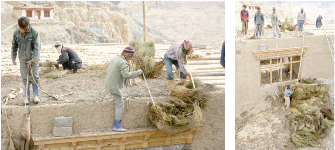
Fig. 11.3 (Left) and Fig. 12.3 (Right) Lamayuru. Ladakh. Yaks is pulled on top of the roof and placed on the wooden subconstruction.
