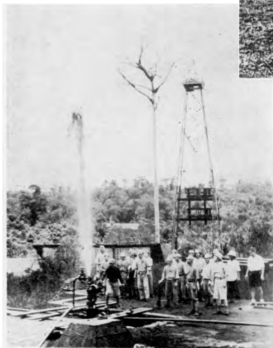
Making Haste with the Restoration Work of the Oil Fields in Balikpapan
