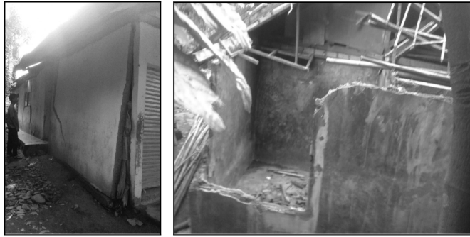
Figure 1. Condition of the roofs and walls of houses due to landslides. (Source: personal documentation).
