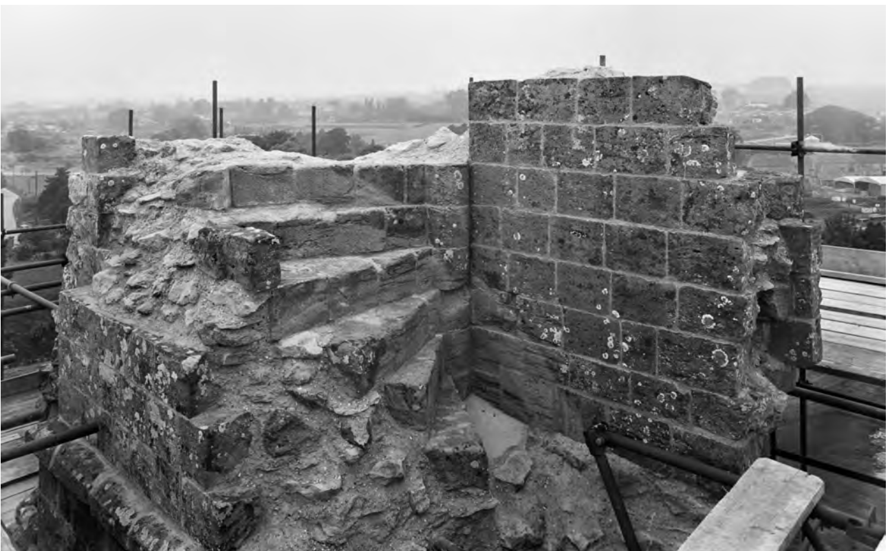
Fig 64 The great tower: the remains of the stairs that rose within the turret above the south-west corner, after consolidation in 1969. Photograph: NMR MPBW A8058/4
