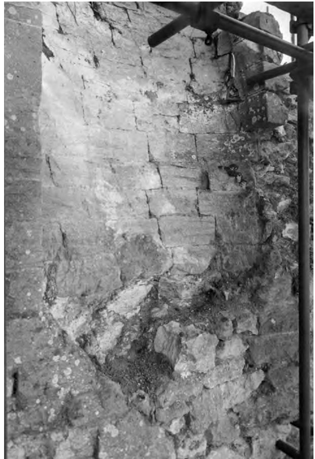
Fig 66 The small tower: detail of the curved ashlar back of the fireplace in the south wall of the chamber at the upper level. Photograph: NMR MPBW A7378/9
