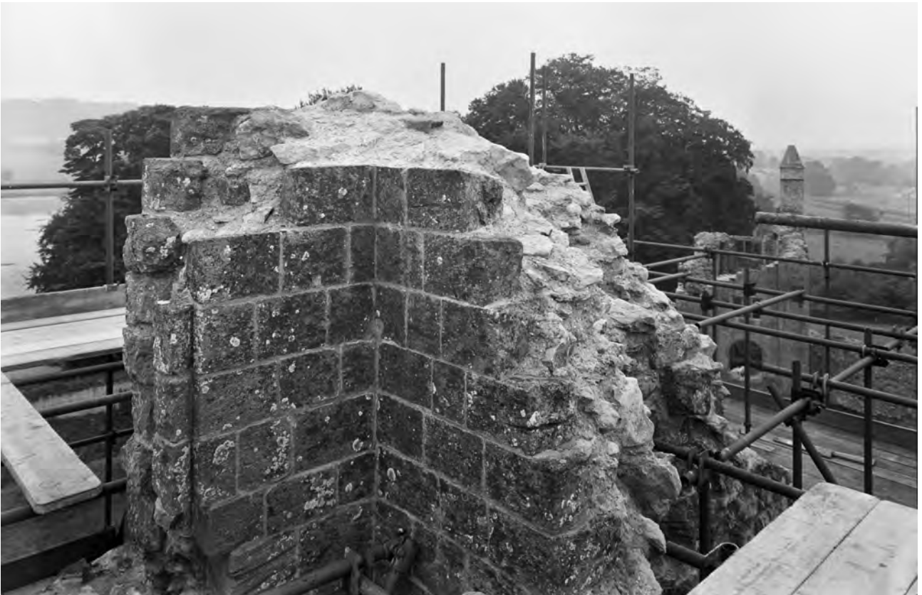
Fig 63 The great tower: the south-west internal corner at roof level showing the base of the parapet turret and, to the left, the remains of the west jamb with the nook shaft of the former doorway leading to the stairs within the turret, after consolidation in 1969. Photograph: NMR MPBW A8058/6
