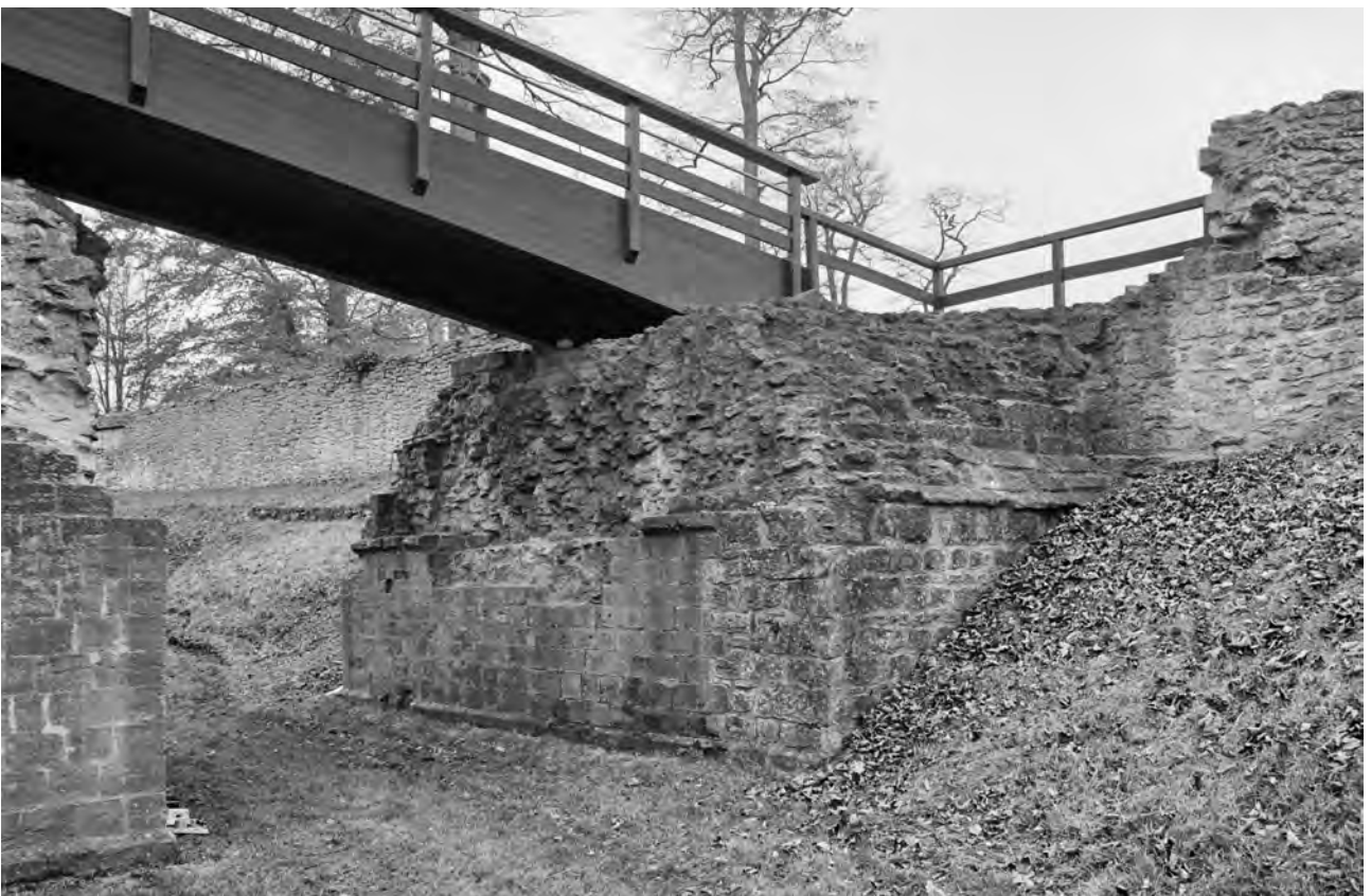
Fig 48 The south-west bridge: the outer abutment to the original bridge with added revetments at each end. Photograph: NMR EH/B925735
