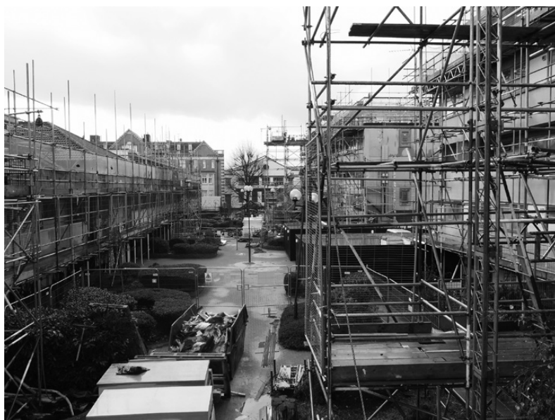
Figure 1.2 New social housing under construction in WALTERTON AND ELGIN COMMUNITY HOMES. January 2018. Image: Pablo Sendra.
