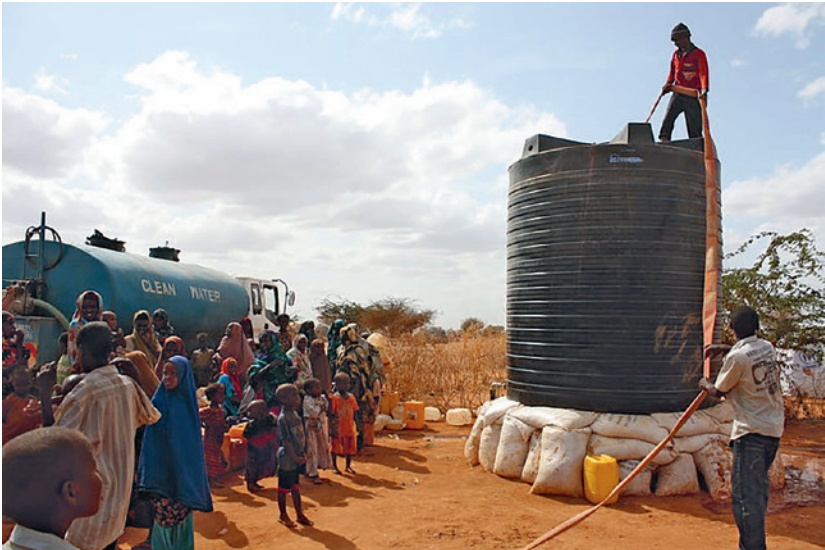
5.5. Installation of an Oxfam water tank, Ifo camp, photo on Wikimedia Commons, July 18, 2011, credited to Oxfam East Africa, Jo Harrison/Oxfam.
