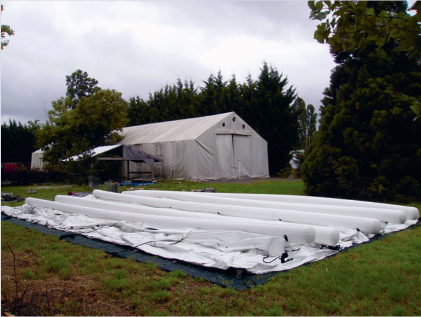
5.11. Inflatable hospital prototype, before inflation process, Mérignac, photo provided by MSF Logistique.
