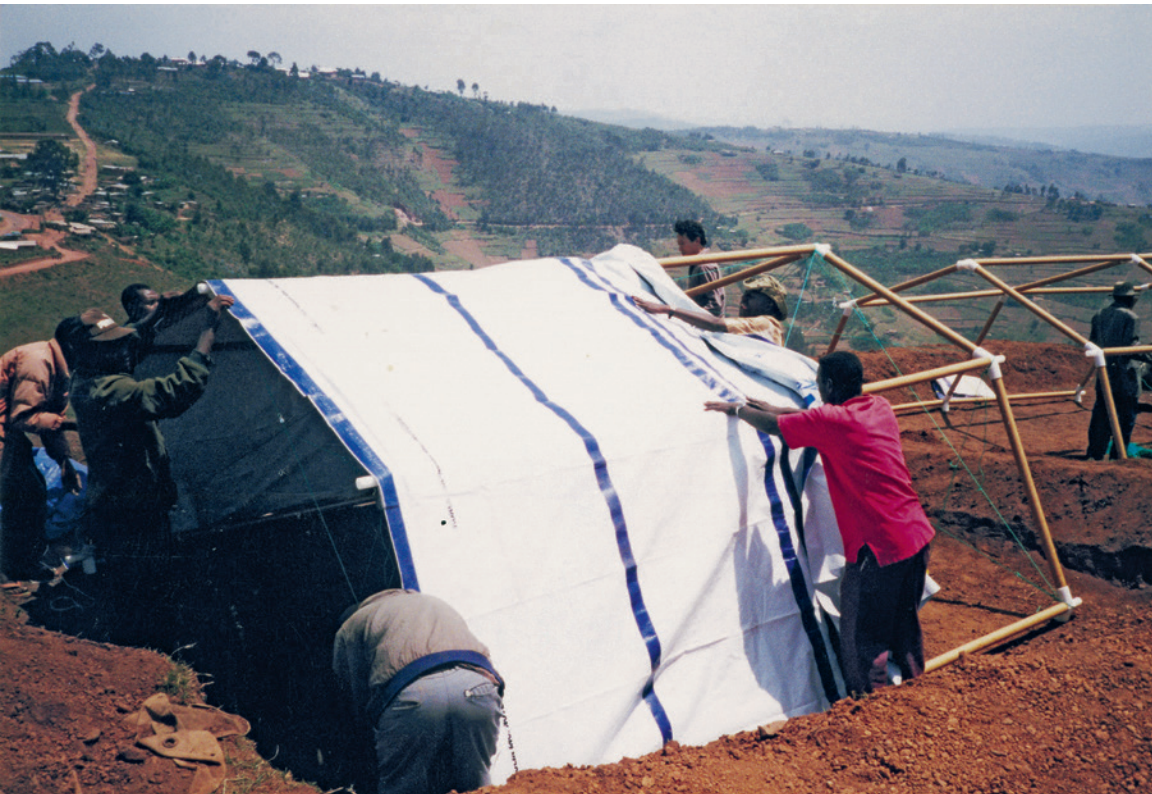
5.1. Shigeru Ban Architects, Paper Emergency Shelters for UNHCR, Byumba Refugee Camp, Rwanda, 1999, © Shigeru Ban Architects.
