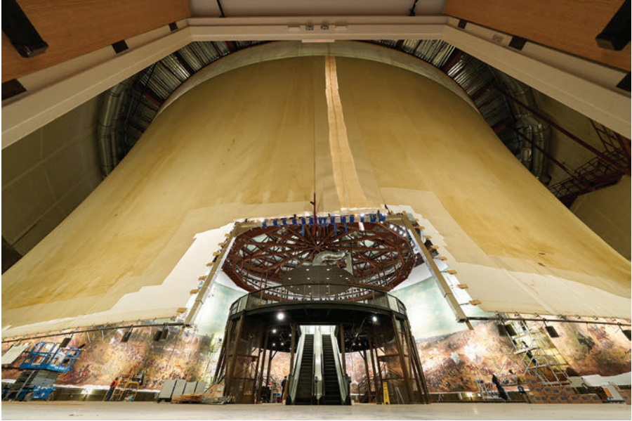
Fig. 6.1. Restoration of the Cyclorama and viewing platform. Courtesy of Atlanta History Center. Photo credit Hales Photography.
