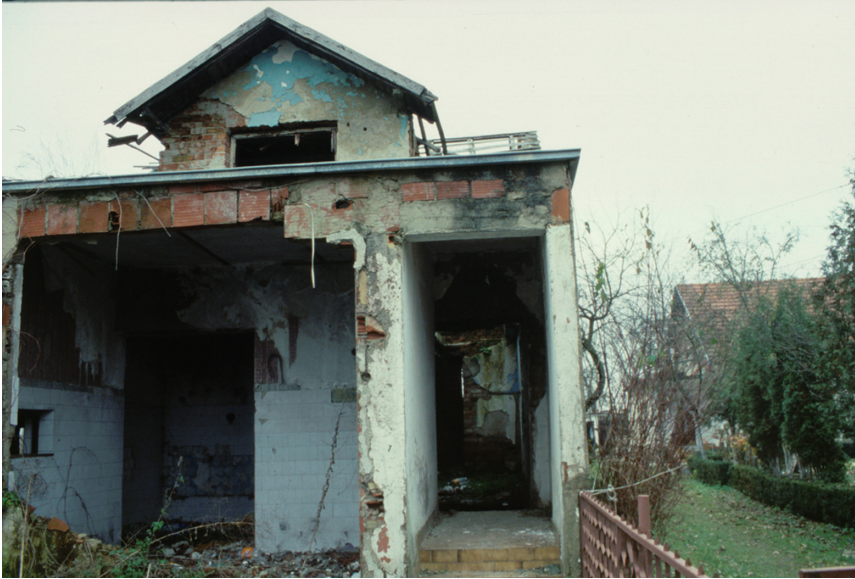
Figure 1.1 A damaged family house near Prijedor in Bosnia-Herzegovina in 2001. A large number of family houses were destroyed in the area in the campaigns of ethnic cleansing between 1992 and 1995. Credit: Laura Huttunen.
