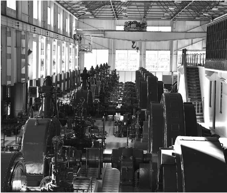
Figure 6.4 Turbines of Waddamana power station, 2021; photograph by author
