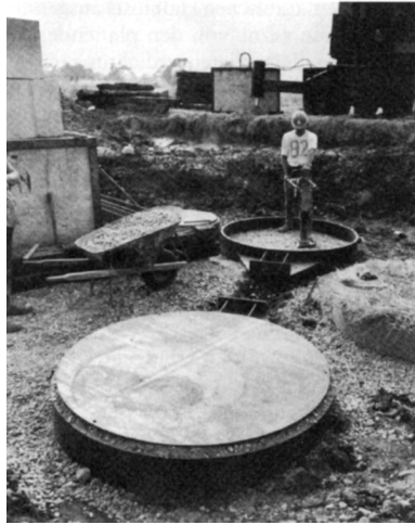
Figure 2.17 Preparation of a horizontal load test on vibro stone columns. (Courtesy of Keller Group plc, London, UK.)
