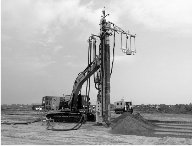
Figure 3.9 Fixed mast crane attachment for head room restrictions with telescopic vibrator extensions and cable tightening device. (Courtesy of Keller Group plc, London, UK.)
