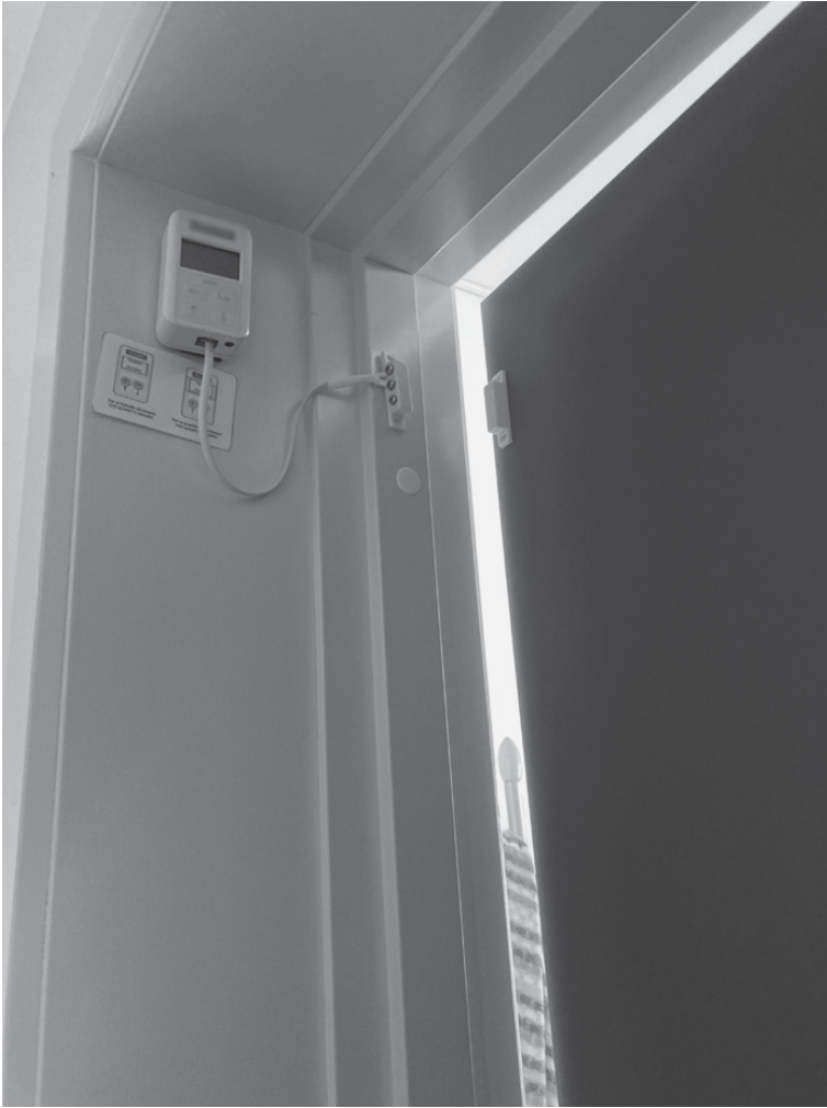
Figure 3.2: A door sensor
