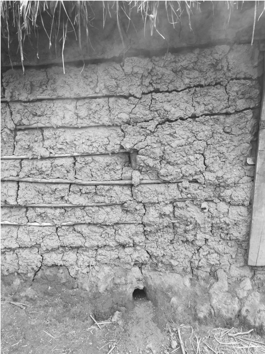
Figure 6.1 Rat tunnel at base of mud-and-dung home in Moramanga District Photograph by Genese Marie Sodikoff, 2017
