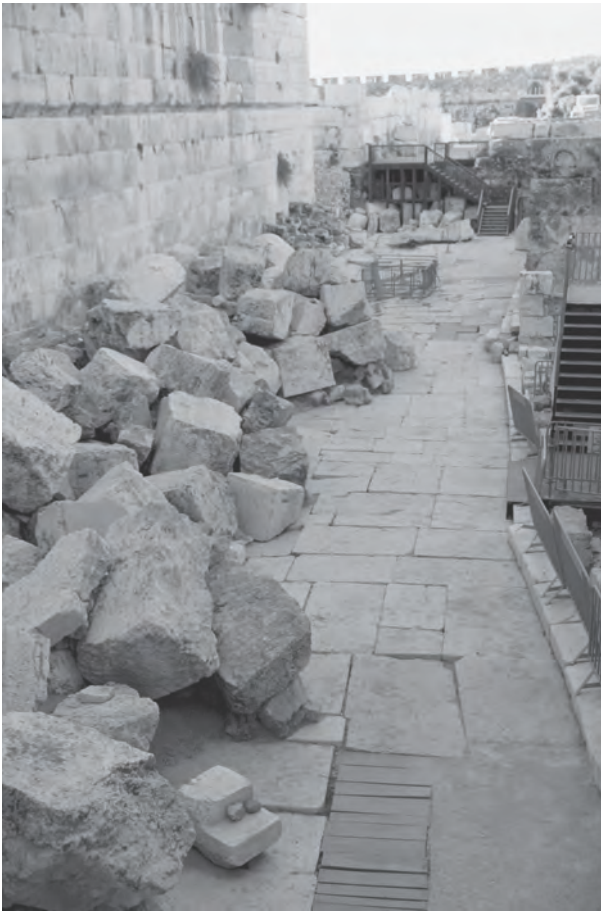
Figure 6.7 The Herodian Street with the collapsed stones. Can millions of visitors go here?
