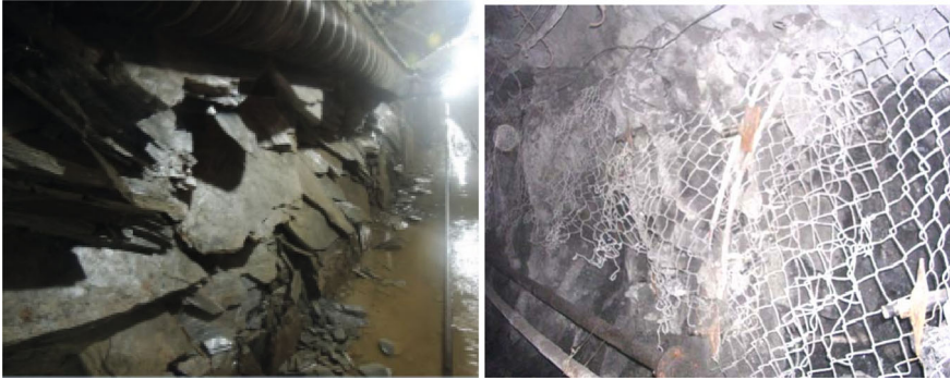
Fig. 5.1 Broken surrounding rock in the mining area
