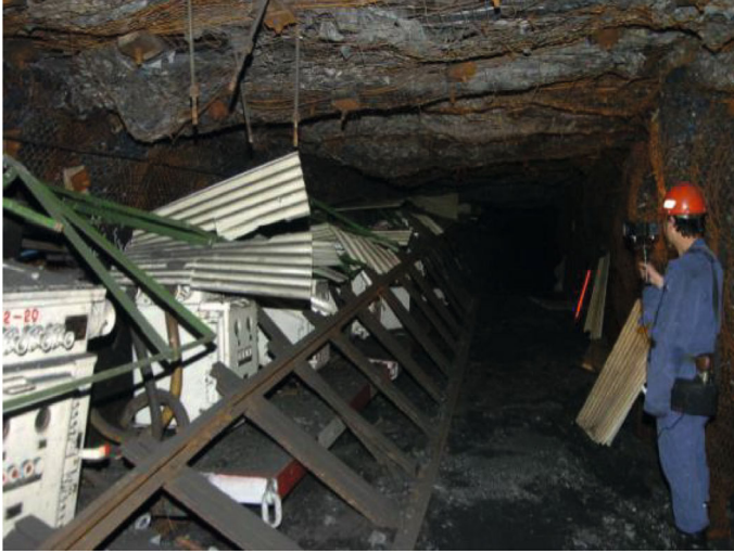
Fig. 1.1 Damage to the roadway after the disaster
