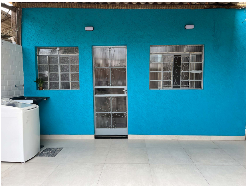
Figure 2.6.6 After condition of a house renovated with Arquitetura na Periferia technical aid. Photo courtesy of Arquitetura na Periferia .
