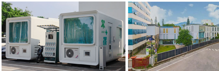
Fig. 7.13 PV future roof DC community DC 48 V storage-swapping research pilot project
