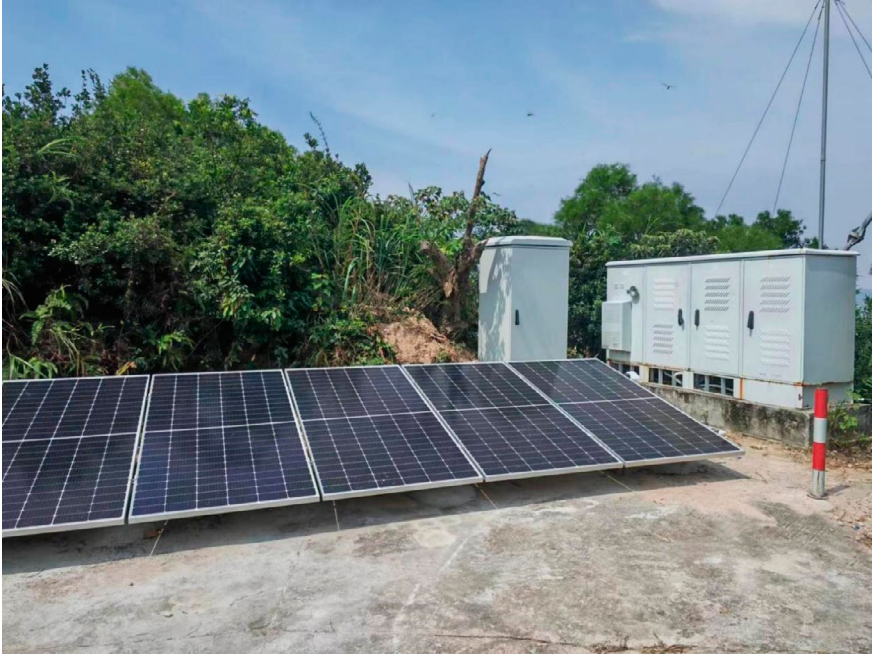
Fig. 7.8 Zhuhai Hebao Island 5G base station
