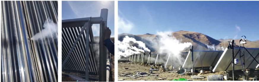
Fig. 7.15 System problems caused by excessive heat in summer
