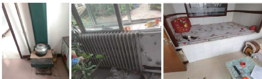
Fig. 3.5 Winter heating facilities for farmer households in a village
