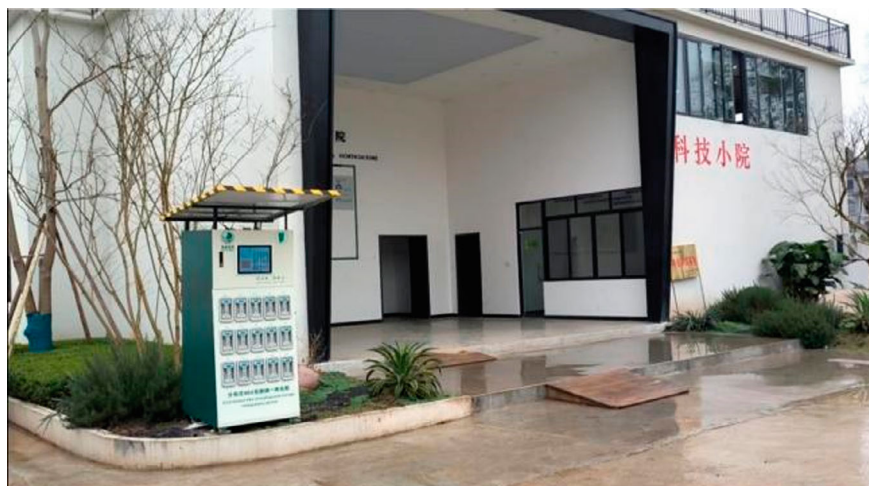
Fig. 7.14 Rural electrification pilot project of State Grid—Chongqing Baihui Park
