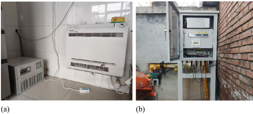
Fig. 7.6 PV-driven air-to-air heat pump system a Air-to-air heat pump indoor unit; b Control system cabinet
