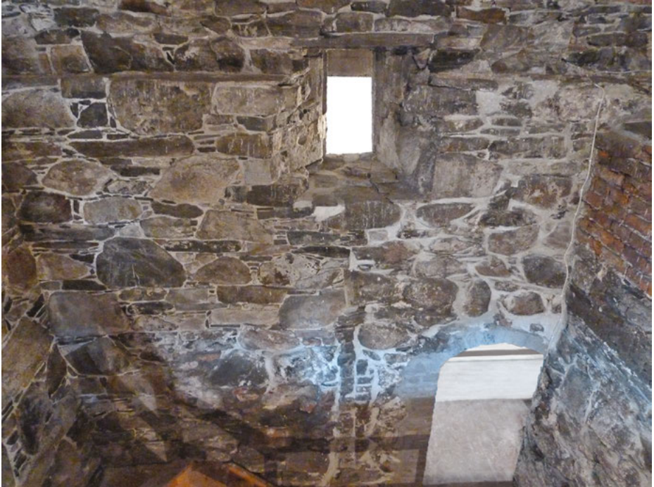
Fig. 7.10: The royal palatium at Holmen. The gate-tower probably built by King Håkon IV. Original internal masonry (south wall). Photo: A. T. Hommedal.
