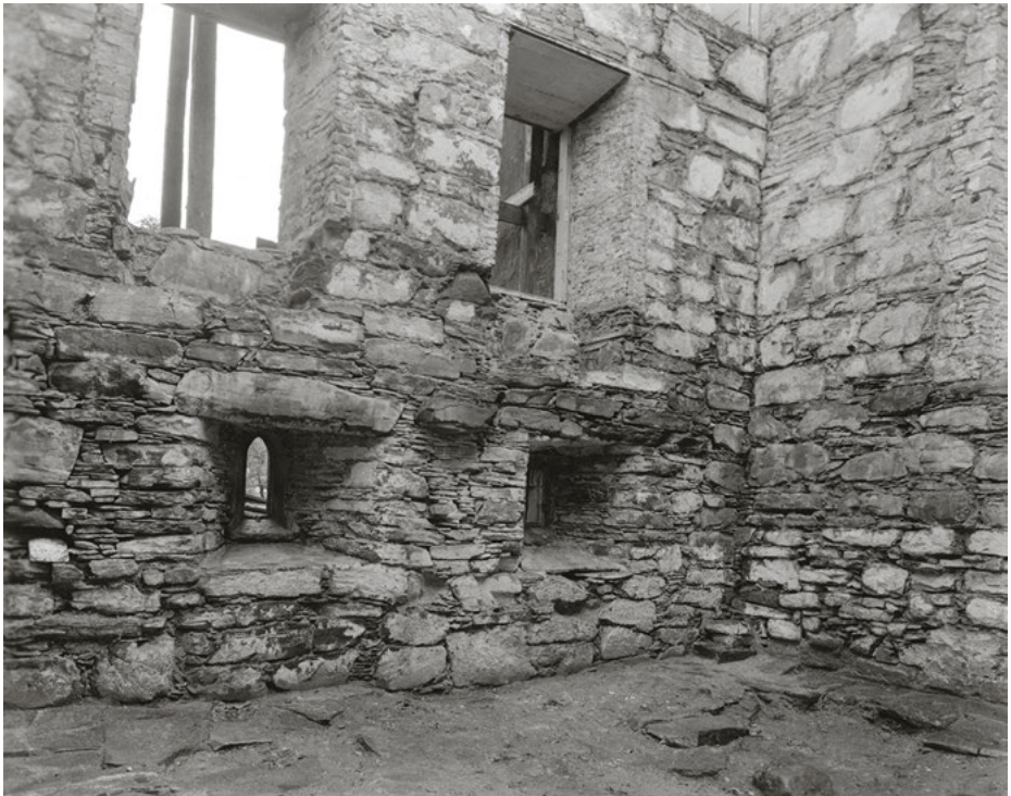
Fig. 7.22: Utstein. The south-eastern part of the possible royal residence, 'G' in Fig. 7.21. In the basement: the original openings for the two pointed windows can be seen. Photo: G. Fischer. Source: The Directorate for Cultural Heritage.
