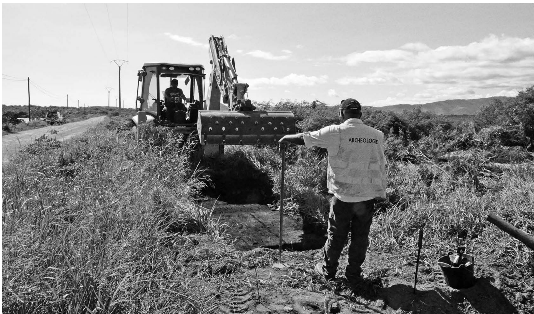
Figure 10.3. The backhoe removing a thin layer of archaeological fill in square SD.14.
