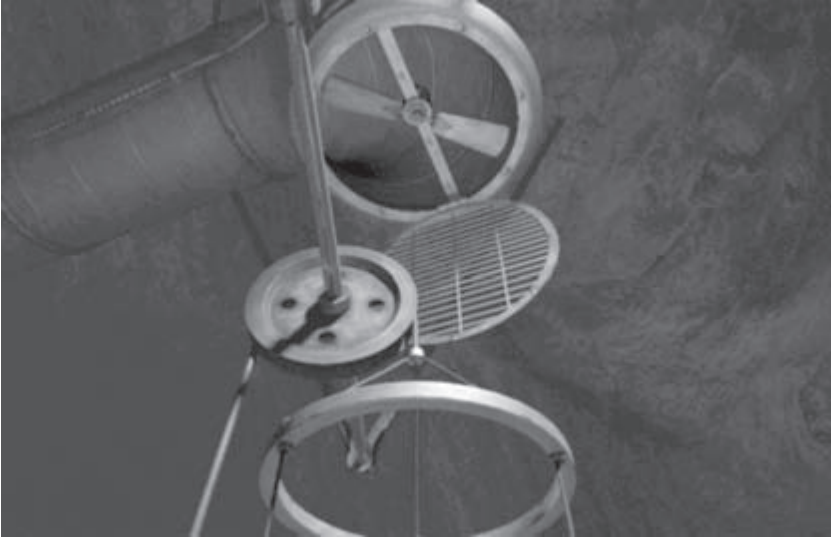
Fig. 19. The air vent does not appear to be big enough to crawl through, but it is.
