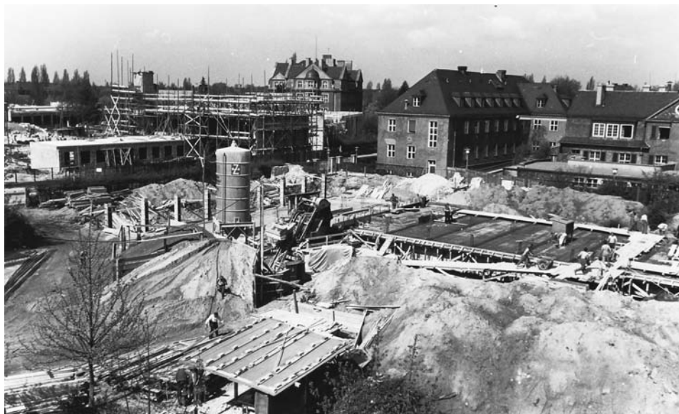
Fig. 4.20. Construction site of the Institute for Electron Microscopy, the library and the administration building, 9 May 1958. In the background on the left, the construction site of the campus of the Freie Universität.
