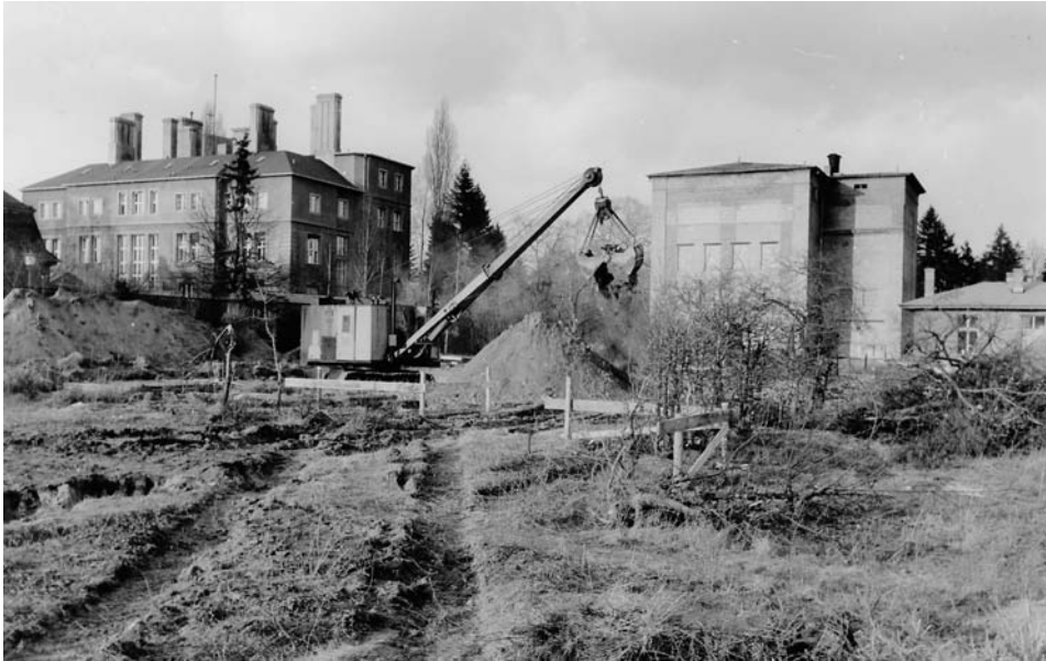
Fig. 4.18. The site being prepared for the construction of the library and administration building, 10 March 1958. On the left, the main building of the FHI. On the right, the Minerva Tower and, far right, the "Radium Hut" of the former KWI for Chemistry.
