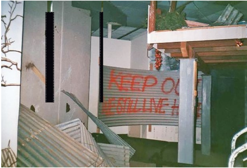
Figure 14: Cyclone damage, 'Cyclone Tracy' exhibition, in 1998.
