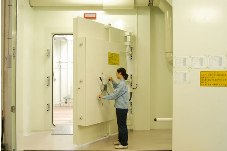
Fig. 4 Fumigation room capable of performing either gas fumigation, carbon dioxide treatment, or low-oxygen treatment
