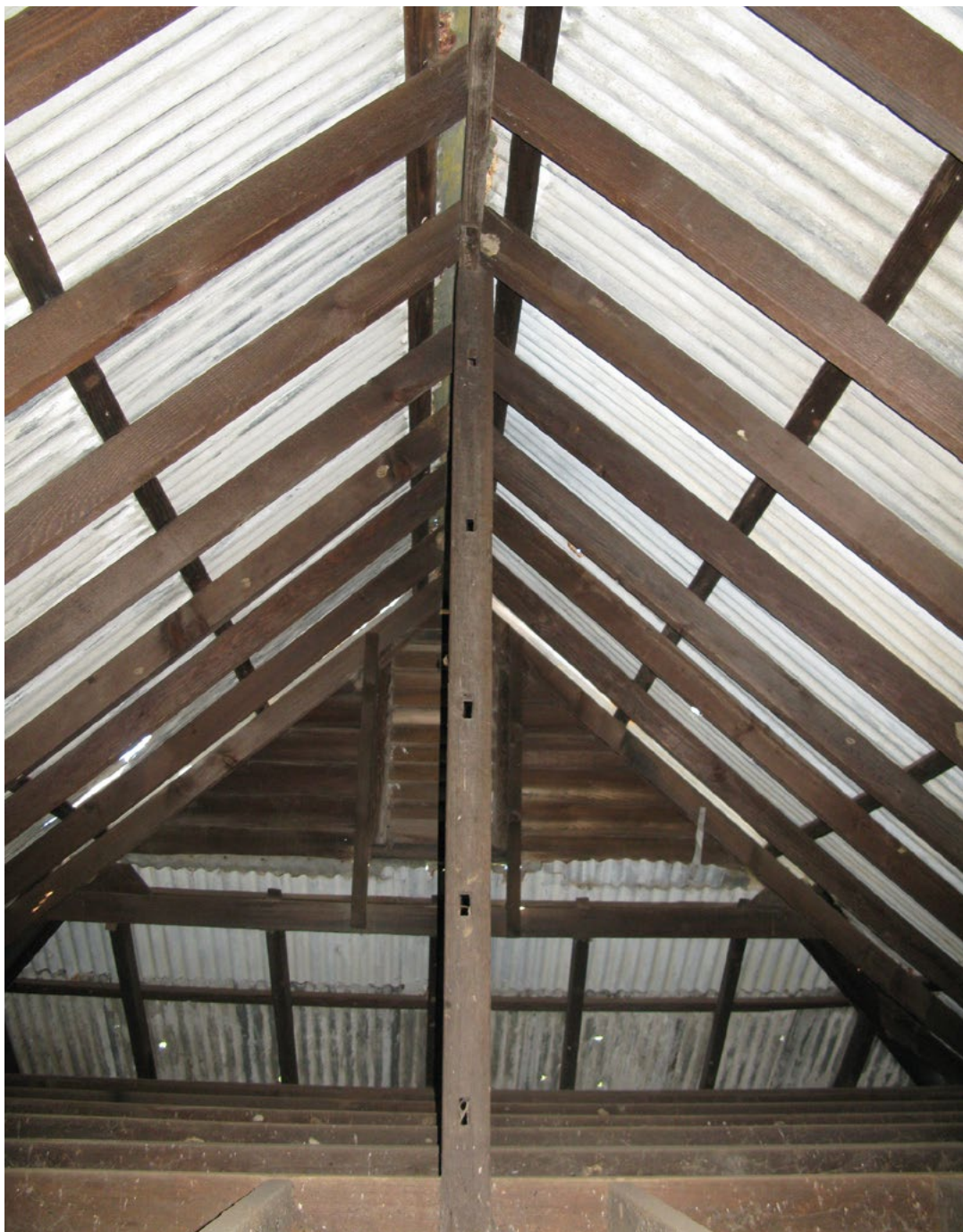
Figure 4.20 Repurposed top-plate used as a roof support pillar, Lenakel church.
