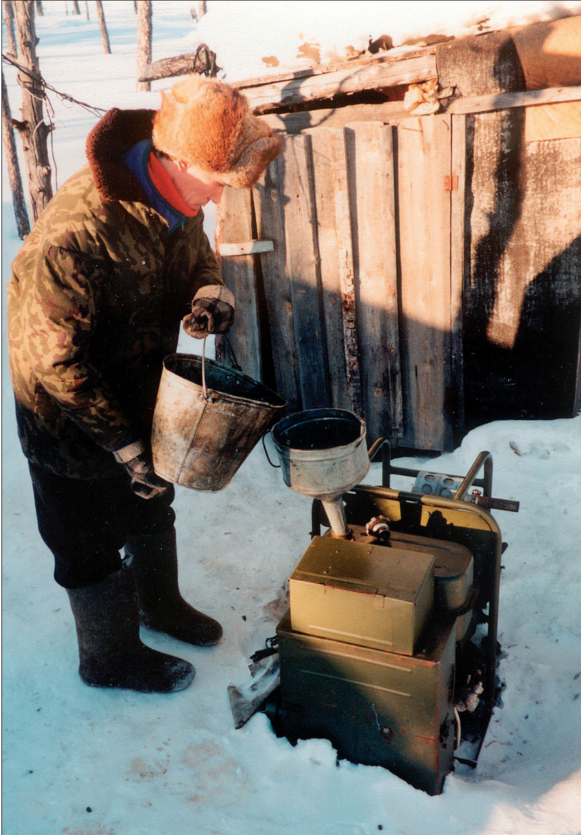
Figure 8. An electricity generator in Yuri Vella's winter camp, 1999.
