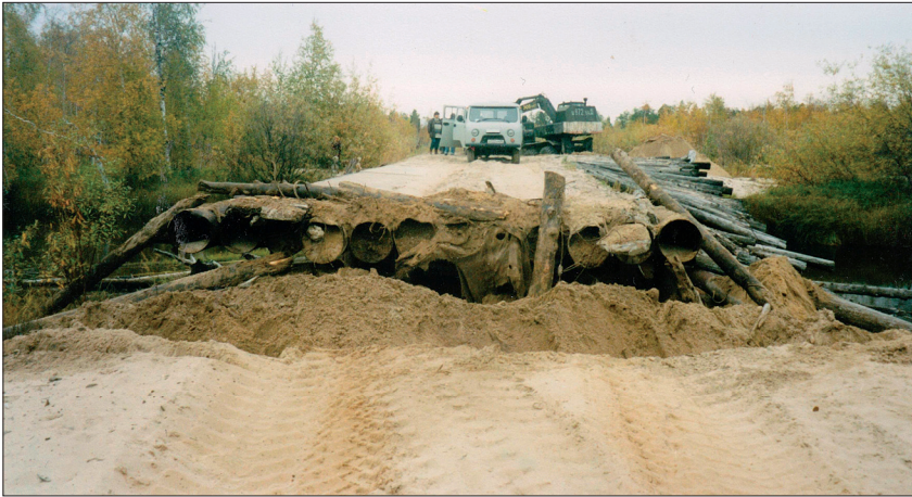
Figure 11. A bridge vital to the natives, destroyed on the orders of Lukoil. September 2000.
