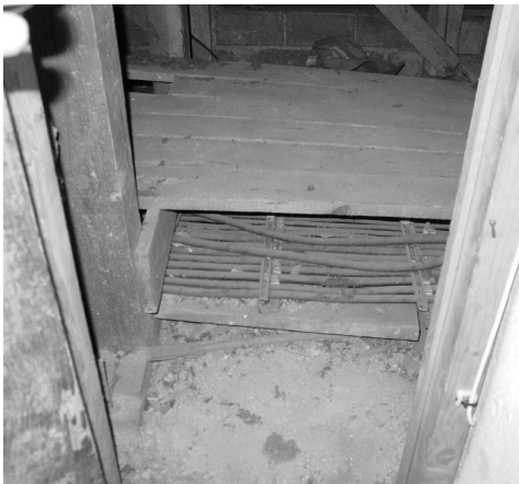
Figure 10: The remains of the cabling system at Kino Světozor. © Ondra Holomek
