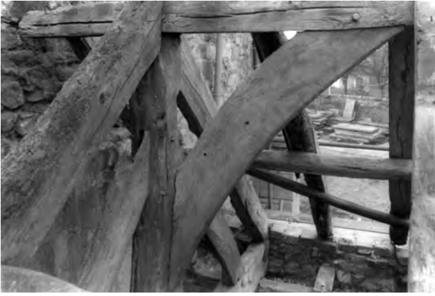
Fig. 555: North porch roof. Detail of the crown-post truss, from the north-east. Photo: Warwick Rodwell
