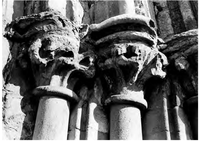
Fig. 95: St Mary's: south porch. Decayed stiff-leaf capitals and abaci on the outer order of the east respond of the arch. Photo: Warwick Rodwell
