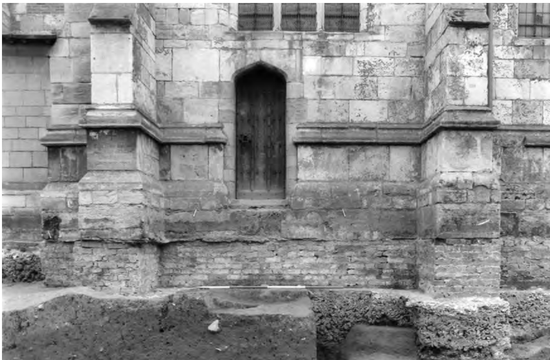
Fig. 619: Organ chamber. Foundations of the north wall (bay 2) during excavation. Scale of 2 m. Photo: Warwick Rodwell
