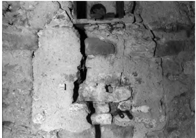
Fig. 418: Tower: Stage 3, west. Infilled double belfry-opening. The three darker rectangular blocks in line near the top are the impost and through-stone. Note also the major vertical crack. Photo: Warwick Rodwell
