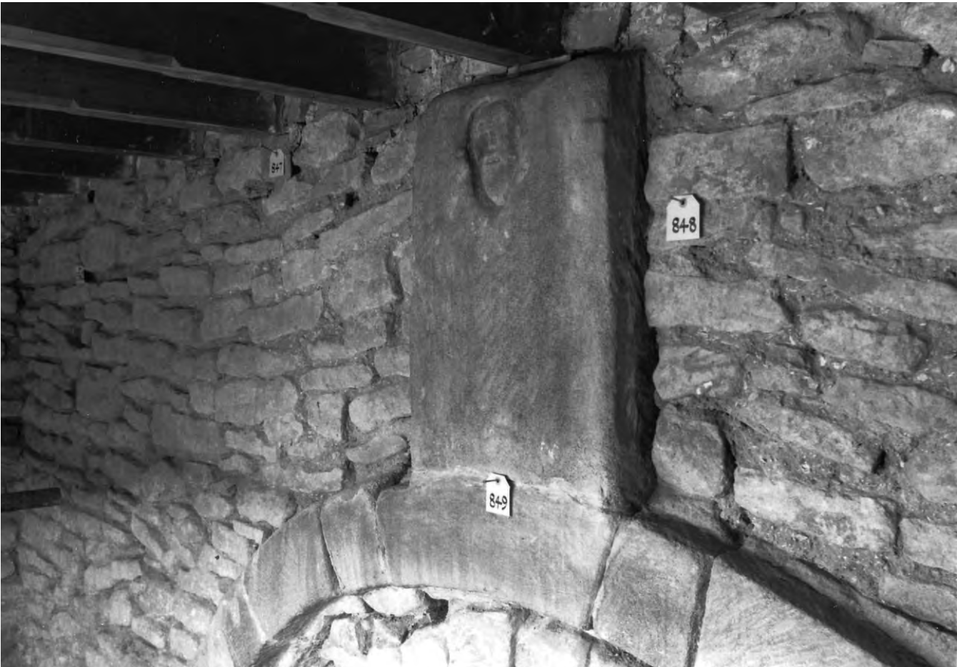
Fig. 309: Tower. 'Humping' of the masonry courses over the eastern arch. View north-east. Photo: Warwick Rodwell
