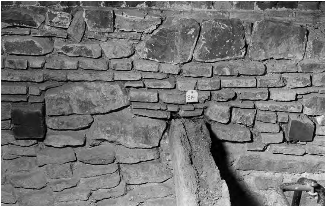
Fig. 329: Western annexe. The top of the north wall, showing one primary floor joist in situ and the stumps of two others that have been sawn off. Photo: Warwick Rodwell
