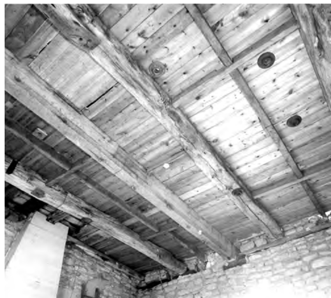
Fig. 295: Tower: floor between Stages 1B and 2. The joists are medieval and later, but the thin spreader-plate in the north wall (right), upon which their ends rest, is primary Anglo-Saxon. Also partly visible on the west side is the casing of the clock pendulum (1852). View north-west, 1983. Photo: English Heritage
