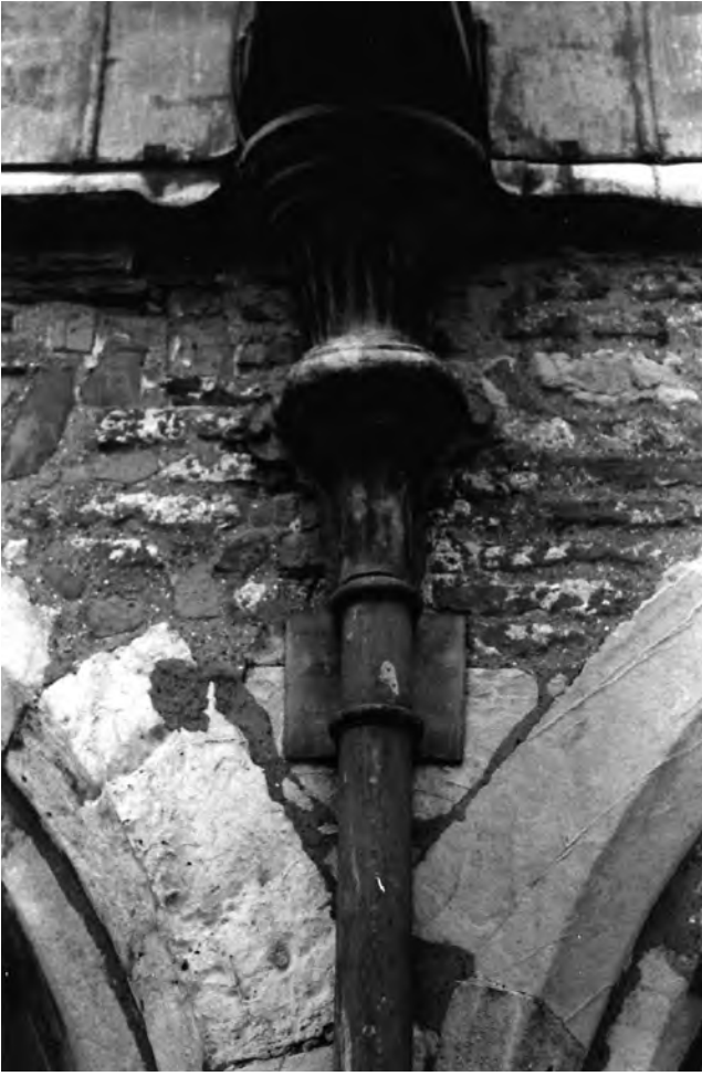
Fig. 585: South clerestory, western rainwater pipe. Fluted lead hopper-head and plain modern downpipe between window bays 8 and 9. Photo: Warwick Rodwell
