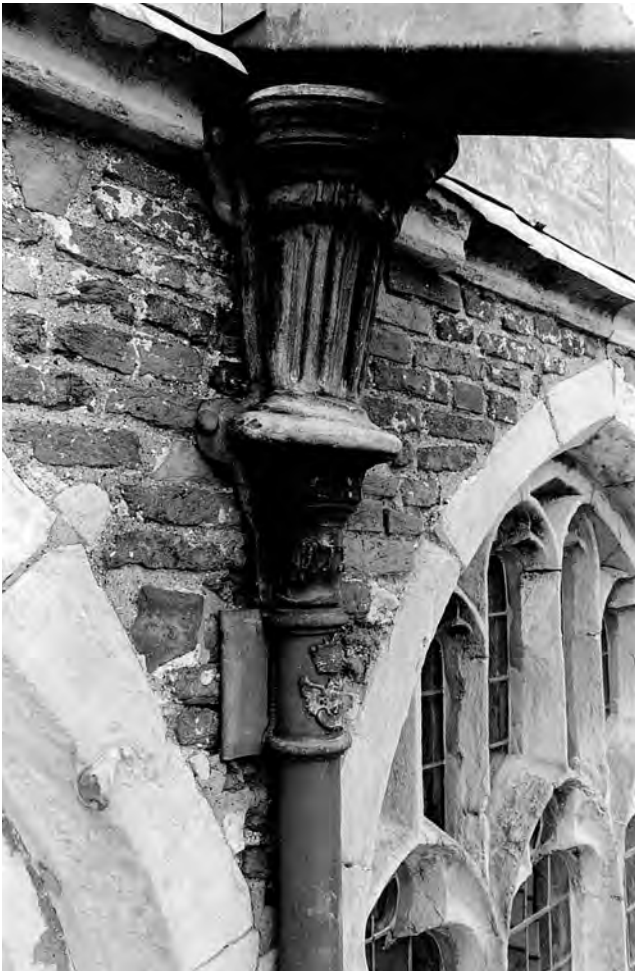
Fig. 583: South clerestory, central rainwater pipe. Inscribed lead hopper-head and decorated downpipe between window bays 4 and 5. Photo: Warwick Rodwell
