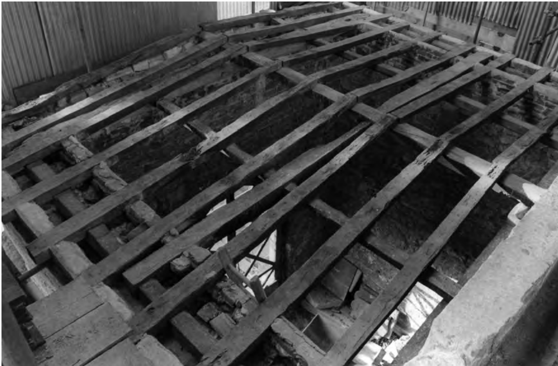
Fig. 546: South porch. View of the roof, from the north-east, after stripping the lead and boarding, 1983. Photo: Warwick Rodwell
