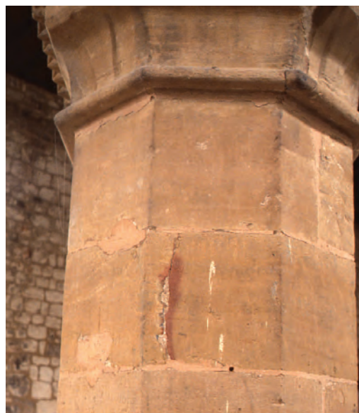
Plate 46: South arcade, pier 1/2. Masonry fracture repaired using hot mastic, and subsequently pointed with lime mortar. Photo: Warwick Rodwell
