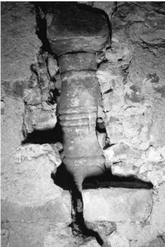
Fig. 313: Tower: Stage 2, interior. Damaged baluster in the blocked western belfry opening. Note also the fracture in the gritstone pad upon which the baluster rests.
