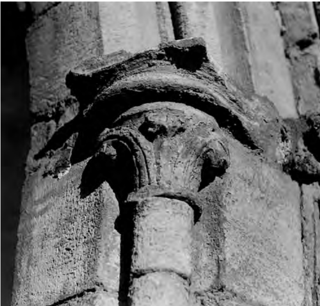
Fig. 94: St Mary's: south porch. Decayed stiff-leaf capital and abacus on the east respond of the innermost order of the arch. Photo: Warwick Rodwell
