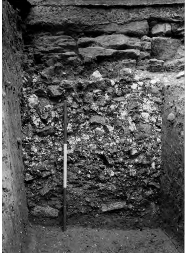
Fig. 303: Western annexe. External face of the rubble foundation on the west side, with the severely fractured limestone plinth course above. Scale of 75 cm. Photo: Warwick Rodwell
