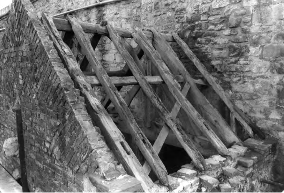
Fig. 553: North porch roof. Viewed from the north-west during repair, 1983. Photo: Warwick Rodwell
