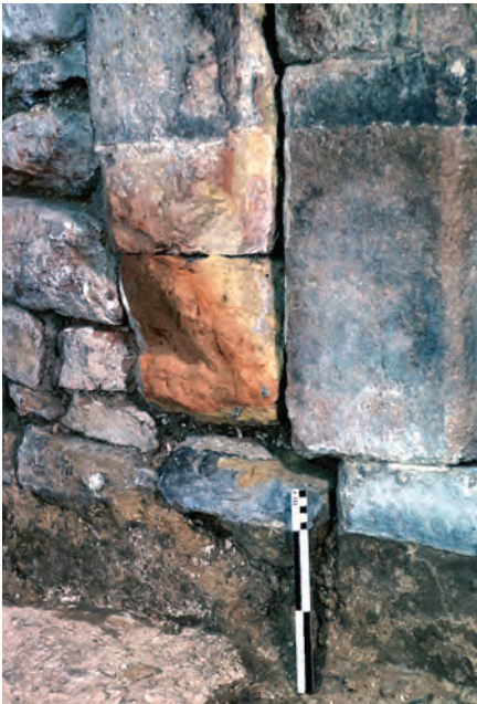
Plate 30: Tower, western arch. The base of the southern pilaster-strip, burnt and shattered by fire. Scale of 25 cm. Photo: Warwick Rodwell
