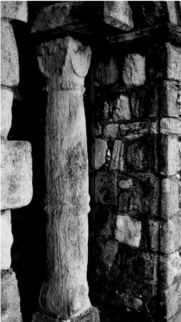
Fig. 413: Tower: Stage 3, north. Mid-wall shaft in the double belfry-opening. View from the north-east, 2005. Photo: Warwick Rodwell
