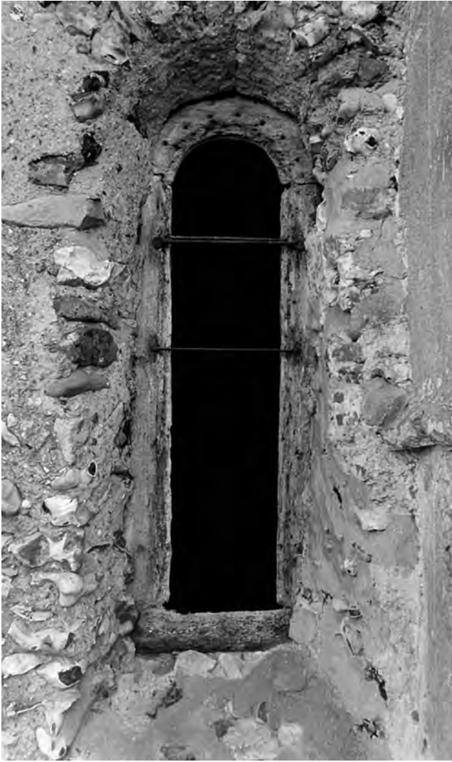
Fig. 331: St Botolph, Hadstock (Essex) . Jointed oak frame of a double-splayed window in the north wall of the nave, integrally built with the flint-rubble masonry. Note also remains of the original lime-render in the reveal and on the external wall face (upper left). Photo: Warwick Rodwell
