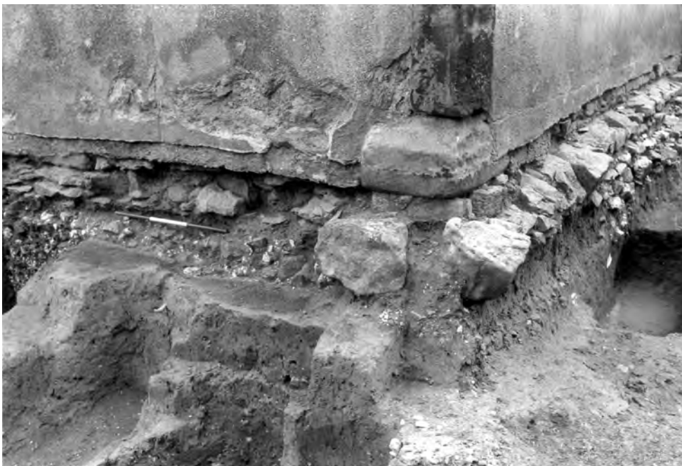
Fig. 326: Western annexe: south-west corner. The limestone plinth running around the base of the walls is present but heavily decayed on the south (right), while on the west (left) it has largely disappeared. Scale of 75 cm. Photo: Warwick Rodwell
