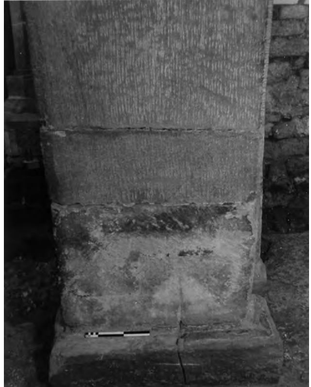
Fig. 281: Tower: Stage 1A, eastern arch. A, north, and B, south responds and bases, showing settlement fractures and Victorian redressing of the masonry (vertical clawing). Scale of 25 cm. Photos: Warwick Rodwell
