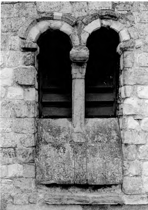
Fig. 409: Tower: Stage 3, east face. Double belfry-opening with later raised sill. Photo: Warwick Rodwell
