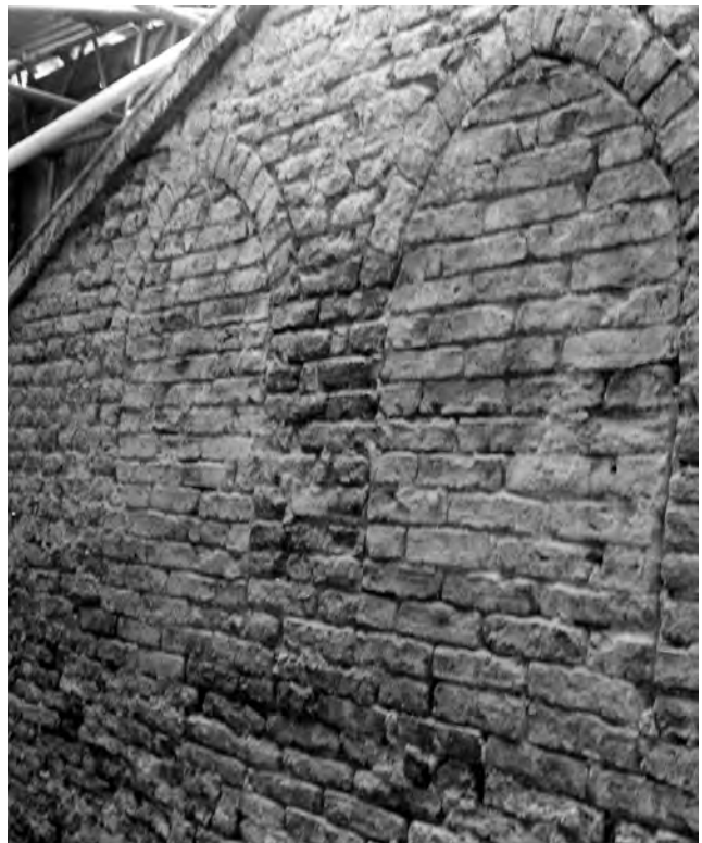
Fig. 590: Nave, exterior of the east gable, 1984. Two blocked openings which formerly ventilated the space between the roof and the ceiling. Photo: Warwick Rodwell
