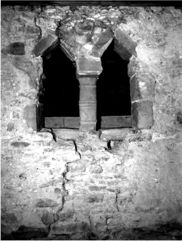
Fig. 299: Tower: Stage 2, interior. East belfry opening, 1983. Note also the cracks in the masonry above and below. Photo: Warwick Rodwell
