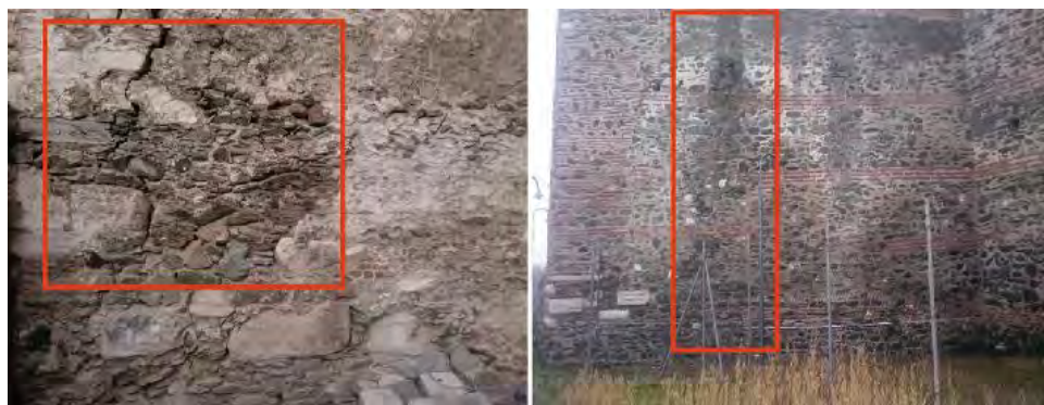
Fig. 4. Visible structural damages (left) and areas of high moisture (right) at various locations of the Heptapyrgion fortress walls.
