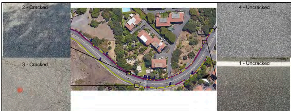
Figure 5. Selection of pavements in different conditions.
