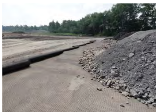
Figure 6. Stabilisation of expressway embankment base constructed from unburnt clay shales – Road 902 project in Gliwice.
