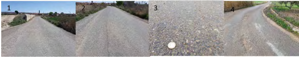
Figure 5. Cement stabilized stretch (1) and WPFA stretch (2) showing a joint. Bituminous treatment integrity (3) and potholes in the joint (4).
