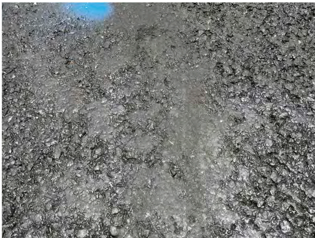
Figure 9. Example of isolated bitumen-rich area of SMA.
