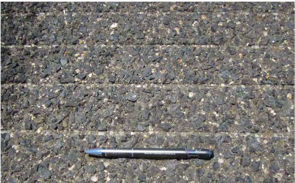
Figure 2. Typical runway surface prior to 2019 resurfacing.
