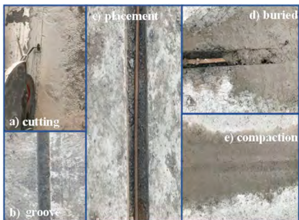
Figure 2. The embedded process of optical fibre sensors in the cement-treated base layer.
