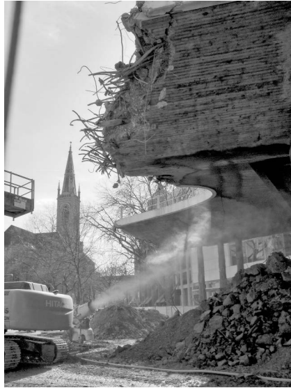
Figure 9: Düsseldorf, Demolition of the ‘Millipede’ next to St. John’s Church (Photo: Perlgrau 2013)
