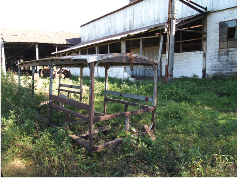
Figure 5.3 Skeletal frame of a railway carriage at the old Puerto Casado tannin factory (Source: author).
