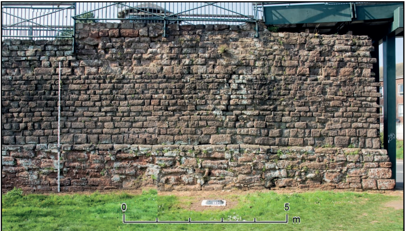
Fig. 6.8 Roman plinth and facework to full height of the City Wall in Quay Lane (photo by Gary Young; © Exeter City Council)
