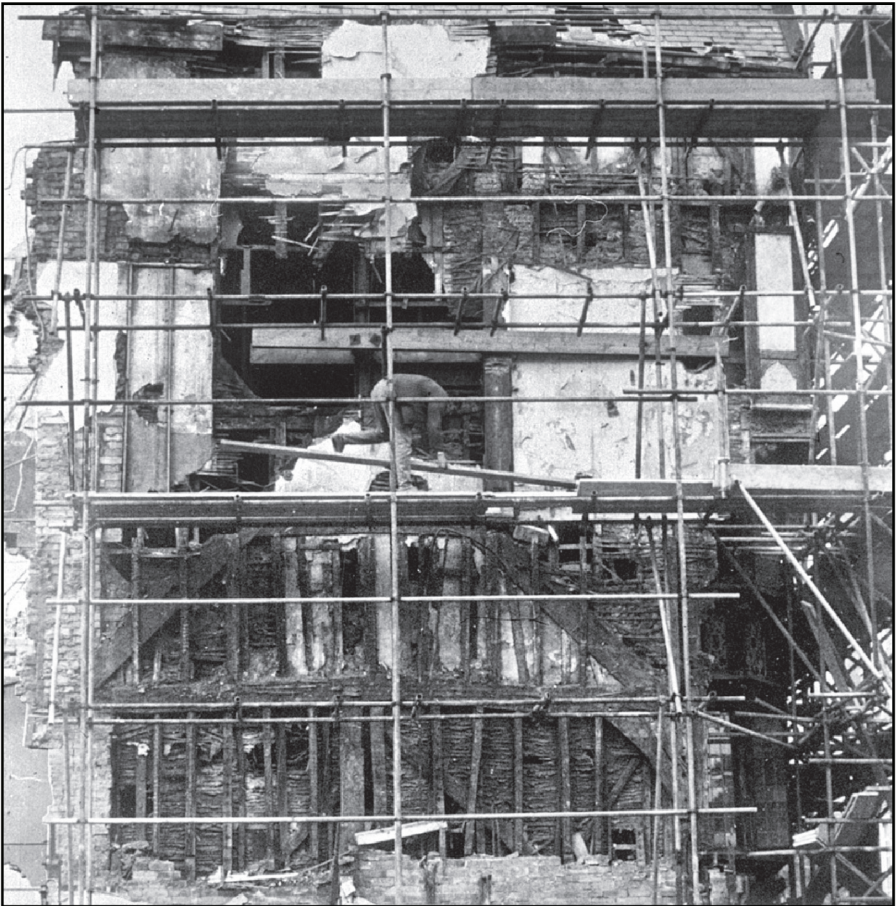
Fig. 8.22 Timber-framed party wall between 224 and 225 High Street, showing the side of the late 16th or early 17th-century house rising above the roofline of a medieval house (photo: Michael Griffiths; © Exeter City Council)
