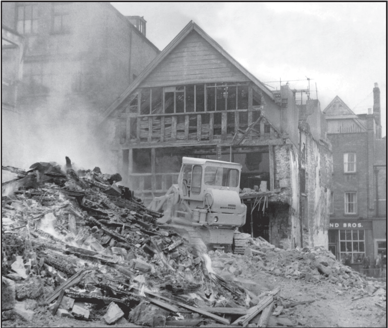
Fig. 1.6 The demolition of 38 North Street in May 1972. For an account of this important building see Thorp 2012 (photo: Nigel Cheffers-Heard; © Exeter City Council)
