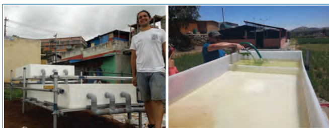
Figure 6.9. Pilot-scale BSP modules of the INNOQUA system installed in India (left) and Peru during inoculation (right).
