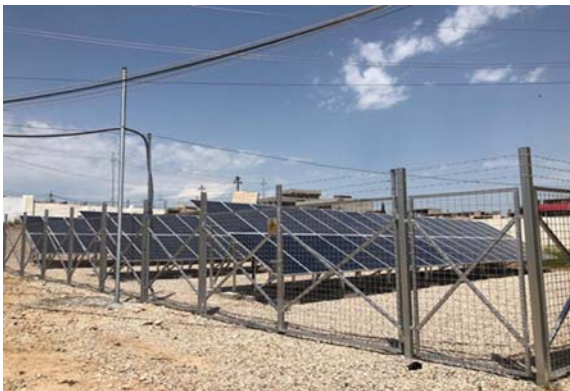
Figure 8.2 Solar-powered water project in Shekhan.
