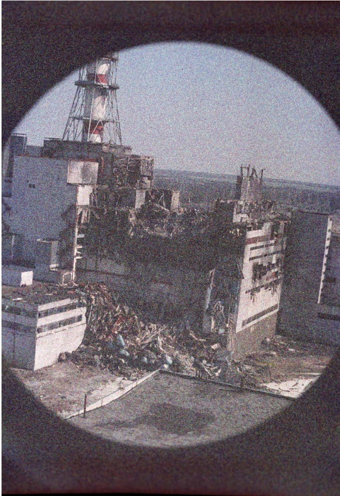
Figure 8.2 Igor Kostin, Aerial photograph of the Chernobyl power plant, April 26, 1986.
