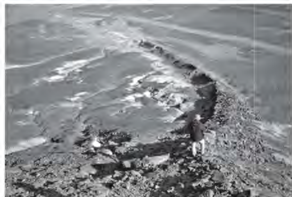
Figure 2.41. The west end of the lower embankment wall CHA003, looking east (CMD 1973).
