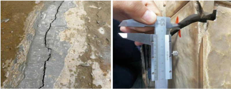
Fig. 9. Cracking of roads and buildings
