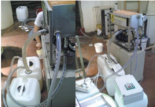
Figure 60: Details of the filter press. Left: detail of the inlet tube, at the left, recognizable by the yellow colour of the Cr(VI) solution at its interior, and the outlet tube of the filter press, white, through which the solution flows after reaction with biomass. Right: panoramic view of the filter press. In foreground the control unit and in the background inlet and outlet tubes of the filter press.
