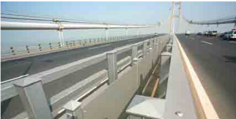
Figure 3: Central stabilizer mounted on the deck of Runyang Bridge
