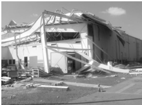
Figure 1. Damage to community center building, Gulfport, Mississippi, following Hurricane Katrina (2005). Photograph by L. T. Phan.
