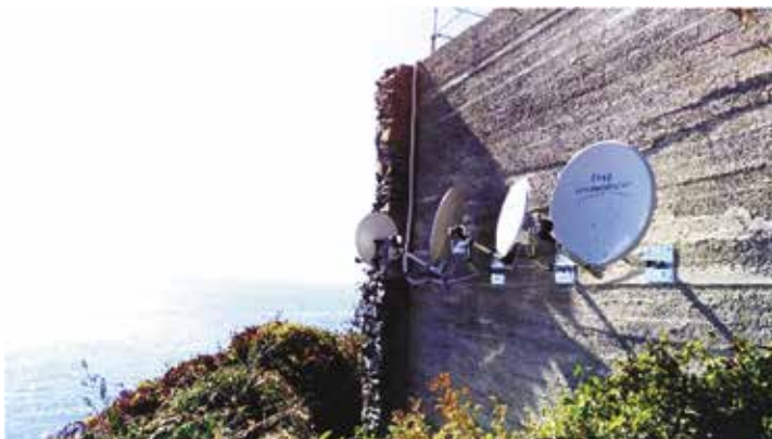
Figure 5 – The four SRS sensor antennas installed on the coast of Corniglia (La Spezia) field site.
