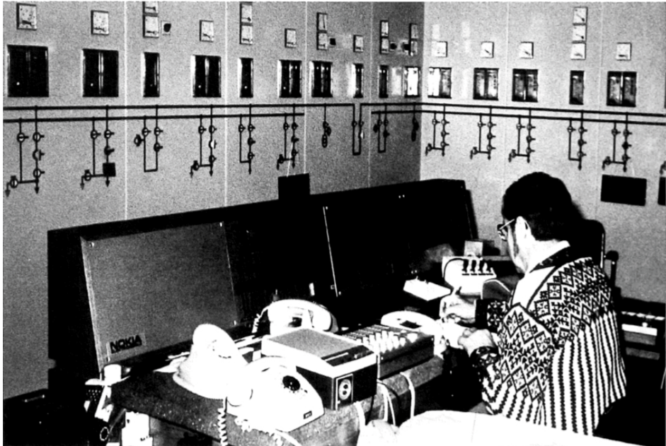
Picture 1. Pekka Kauppinen, Chief Operating Officer of the electrical substation operating VII sa in physical form in the 70's. (located in Viirinkangas)
