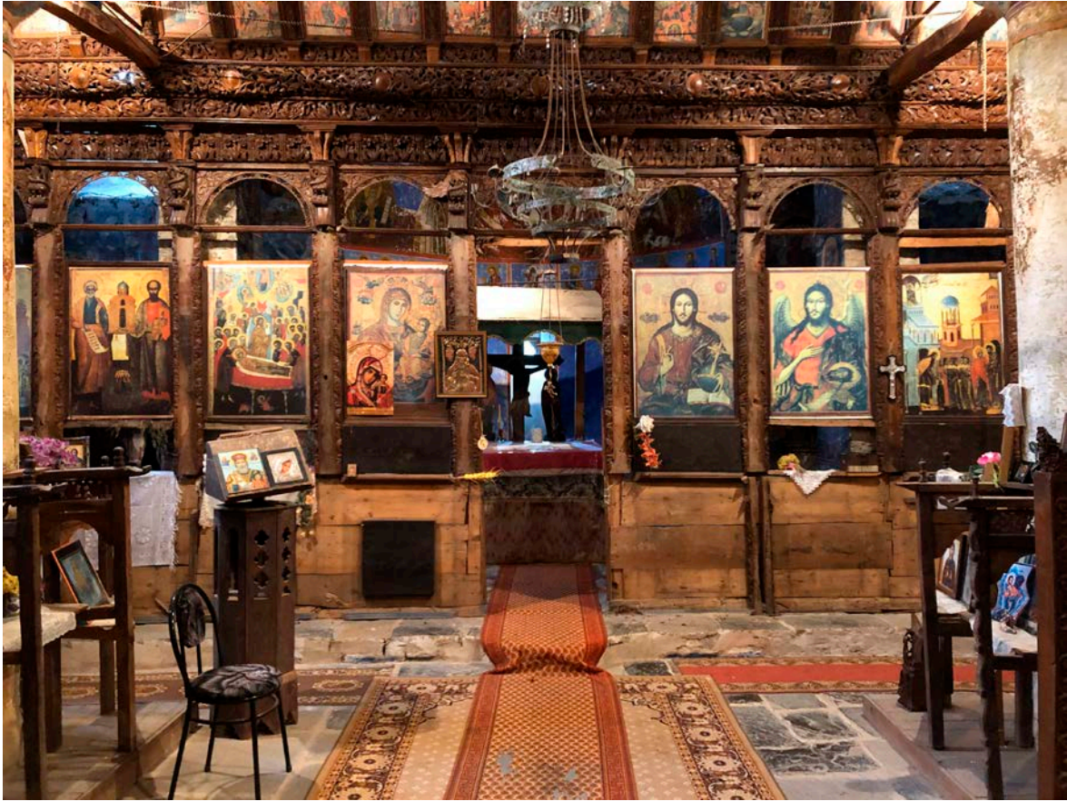
Figure I-5.3.2 View of the carved wooden iconostasis of the church. Significant portions of it have been removed or seriously damaged.
