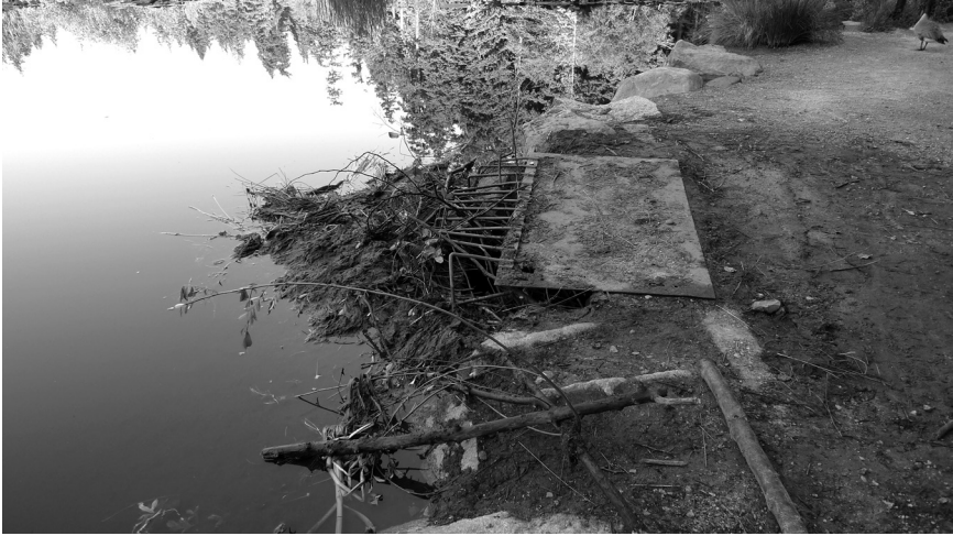
5.8 Beaver Lake's culvert, unplugged. Photograph by Tobias Slezak.
