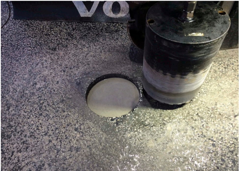
Figure 4. After drilling the cooling water did not drain through the unbound base.
