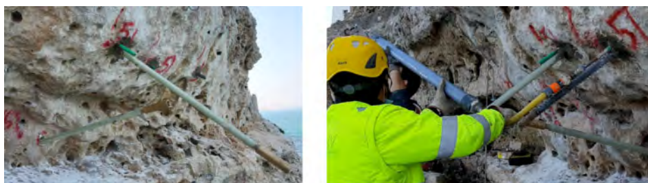
Figure 7. a) VTR bars blocked by Lampocem before injection; b) injection of MasterEmaco 222 through injection tube in CG.
