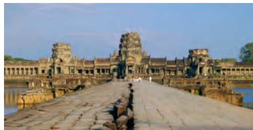
Figure 19. Retaining wall structure of the west causeway of Angkor Wat (south side).
