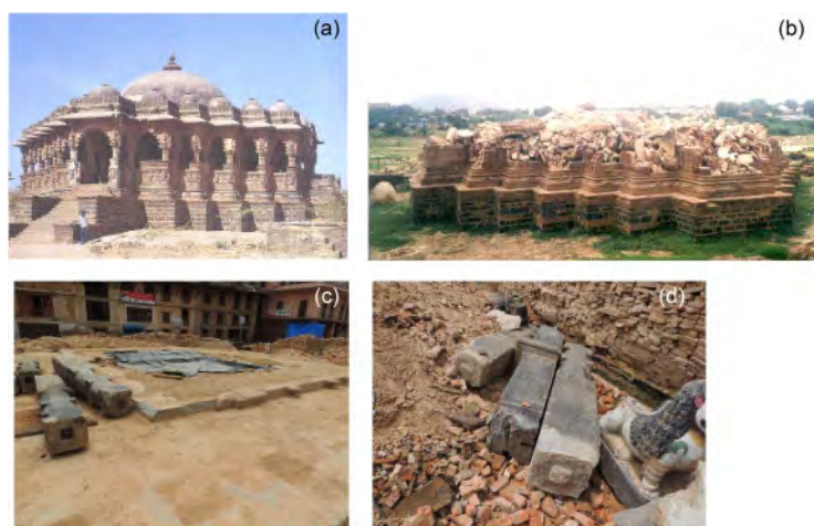
Figure 2. (a)-(b) Observed collapse in historical mandapa Rao Lakha Chattri in Gujarat (Bhuj, 2001) and (c)-(d) Collapse in a stone mandapa in Nepal (2015) with significant tenon-mortise joints.
