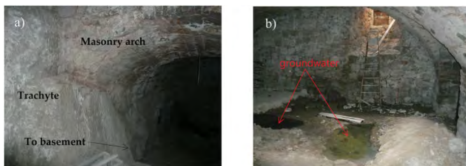
Figure 4. The basement: trachyte outcropping at the entrance (a); groundwater emerging from the floor (b).
