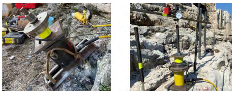
Figure 11. a) Pull test with 1000 kN capacity Hallow piston; b) pull test with 300 kN capacity hallow piston.
