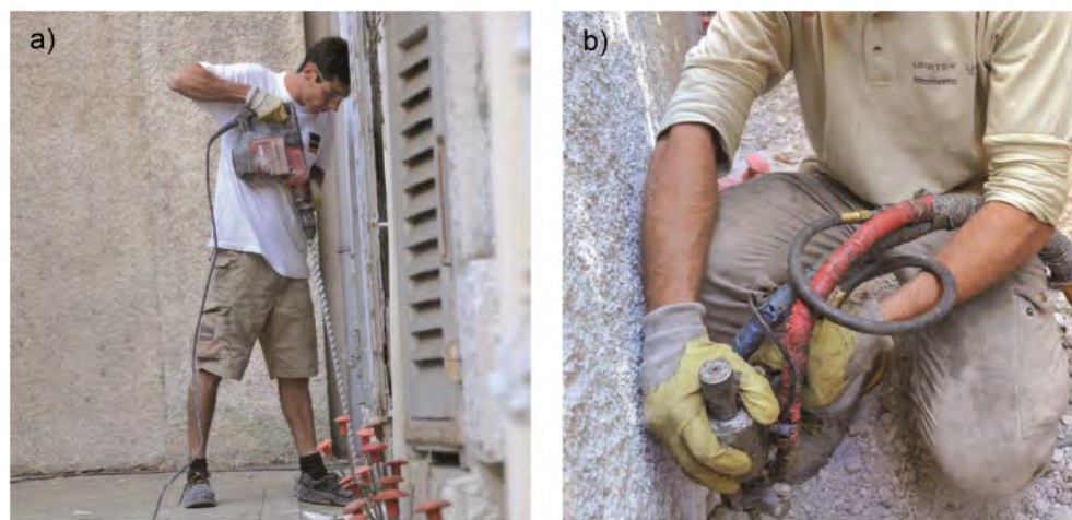
Figure 1. Example of operations: a) Drilling of the borehole; b) Equipment for the injection of the expanding polyurethane resin.
