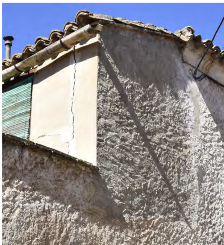
Figure 9. Crack due to the separation of the walls, probably caused by the erosion of the subsoil in Torres de Berellen.
