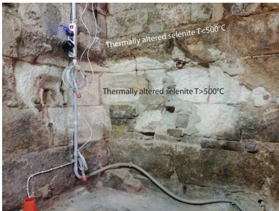
Figure 1. Different degrees of thermal alteration of the selenite rock in the southwestern corner of the Garisenda tower entrance room. Note the recession of the slab surface affected by higher temperature.
