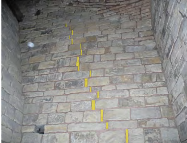
Figure 4. Transversal partition wall above the scarsella; the crack (in yellow) sealed by vertical plates is visible; the extrados of the dome can be seen on the left.
