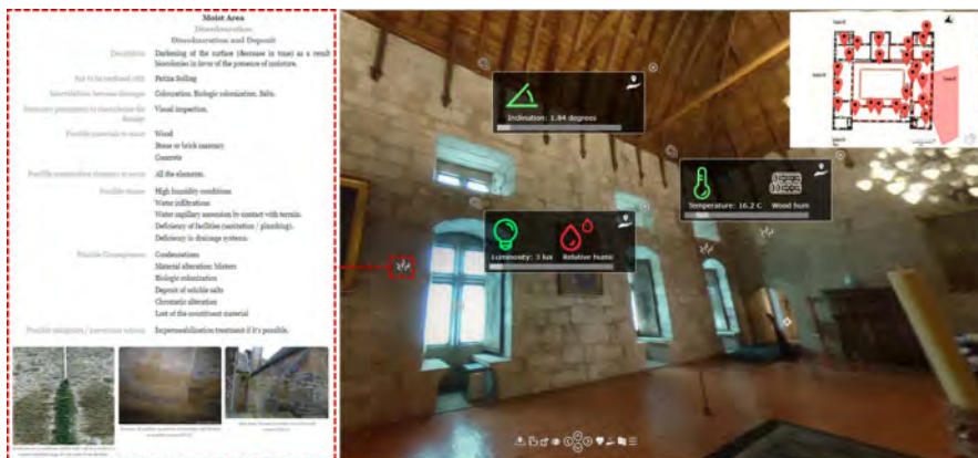
Figure 8. Virtual tour enriched with sensors and damage hotspots, linked to recent acquisition and damage report, respectively.
