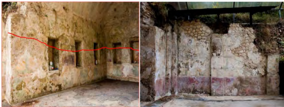
Figure 12. Cracks along the vaulted room (a) and rotated walls in the outer space (b) of the nymphaeum.
