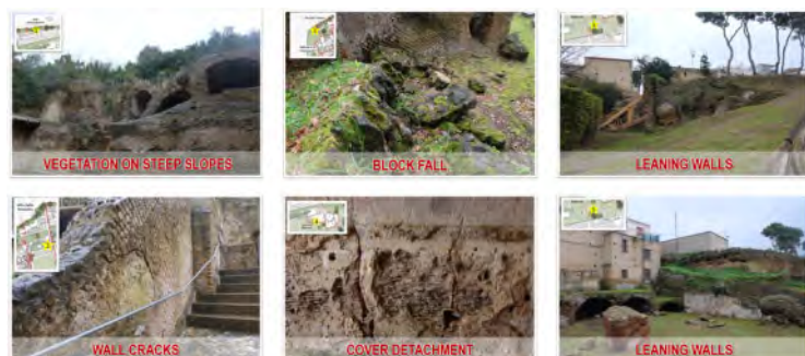
Figure 7. Main typologies of critical conditions surveyed in the site.
