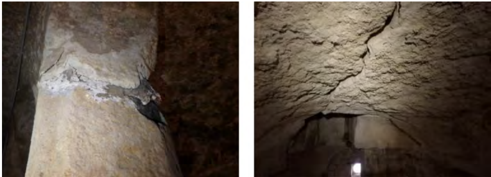
Figure 5. (a) Chipping of the reinforced concrete pillars of the Triforium (left) and (b) Crack in the north Aisle with outcrop (right).
