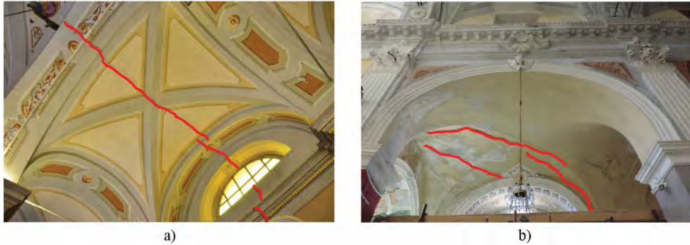
Figure 7. Damage in the vaults: a) cracks continuous between vault and supporting wall, b) multiple parallel diagonal cracks.
