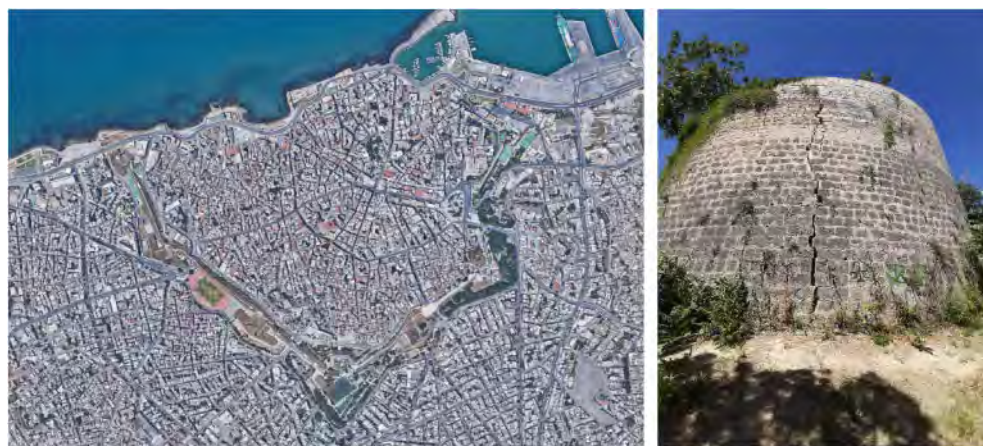
Figure 1. (a) A satellite image of the Heraklion City bastion fortification system (Google Earth). (b) A view of the Martinengo bastion, damaged by vertical cracks.
