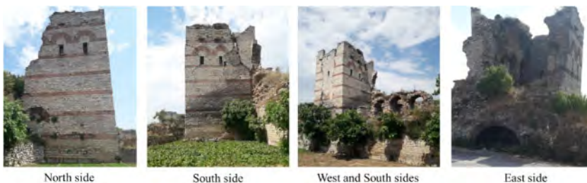
Figure 40. Recent views of all sides of tower 19. The damages caused by 1999 Kocaeli earthquake are clearly visible.
