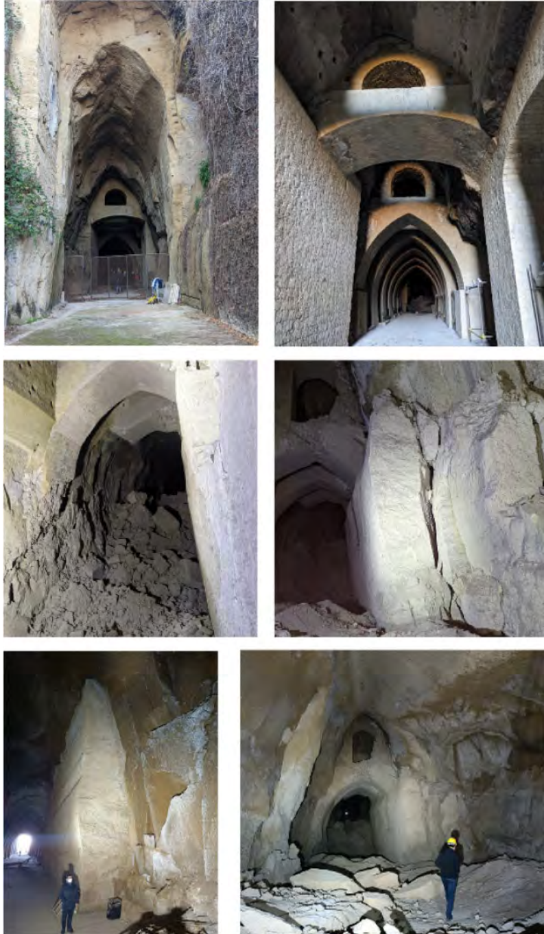
Figure 30. From top left: pictures from the eastern entrance till ca. progressive 150 m. Masonry arches well preserved in the first part, with complete collapse of side walls in the final part. Large subvertical rectangular blocks sometimes on the verge of instability failure.
