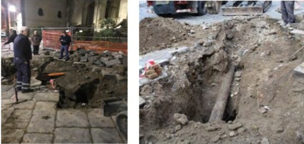
Figure 23. Evidence of damaged pipes of the sewer system of the Incurabili complex.
