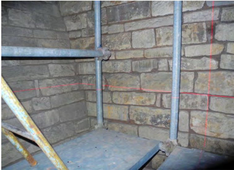
Figure 6. Detail of a partition wall (right) and the extrados of the dome (left) of the Baptistery; the intersection between the vertical and horizontal red lines of the laser highlight the part of the partition wall with masonry in inclined rows perfectly connected with those of the dome.
