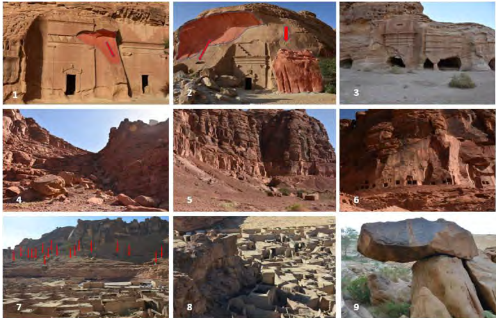
Figure 10. Example of the main instability processes affecting the different archaeological sites belonging to AIUla region: 1&2 rock slide and free fall in Hegra; 3 basal erosion affecting pillars and rock facades in Hegra; 4&5 rock blocks fallen in Dadan; 6 condition of rock cliff affecting the Lions tomb in Dadan; 7 rock blocks accumulation in AIUla Old town western cliff; 8 potential slope instability inside AIUla Old town; 9 unstable and fractured rock arts block in Jabal Ikma.
