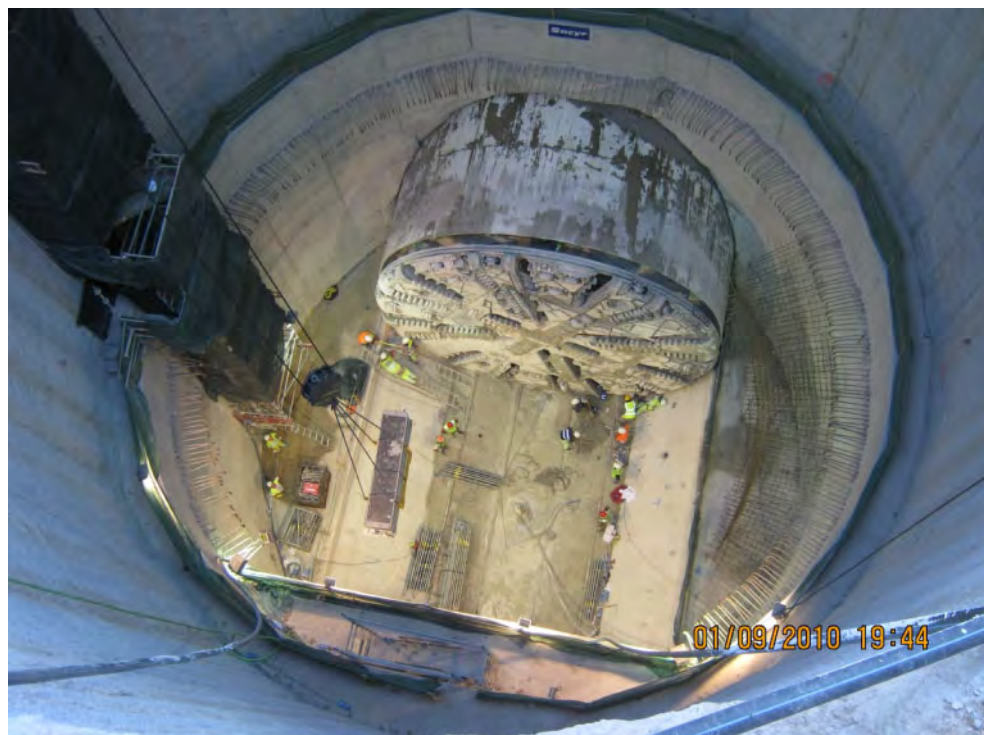
Figure 33. Photograph of the Padilla shaft and the head of the EPB Shield, before approaching the Sagrada Familia Temple.
