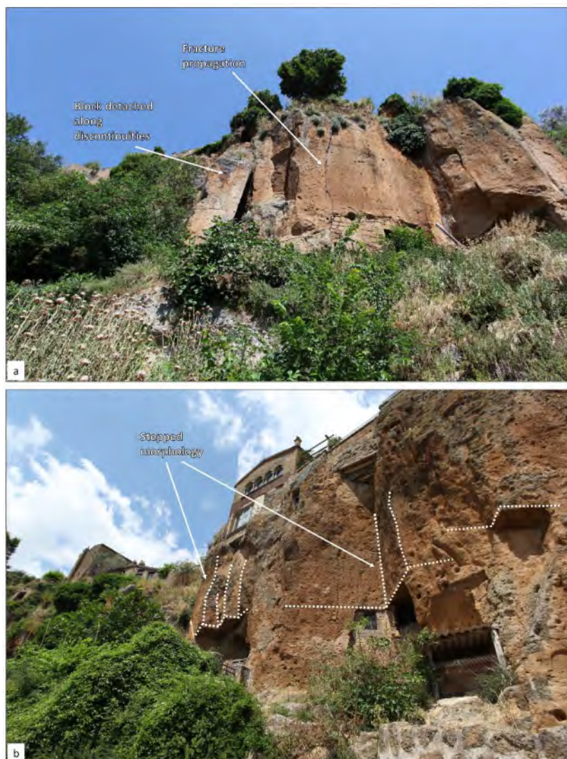
Figure 9. Overview of the processes affecting the evolution of the upper cliff. a: View of the southern cliff displaying fracture propagation and structurally controlled block detachments. b: Example of stepped morphology frequently observed within the massive ignimbrite deposit.
