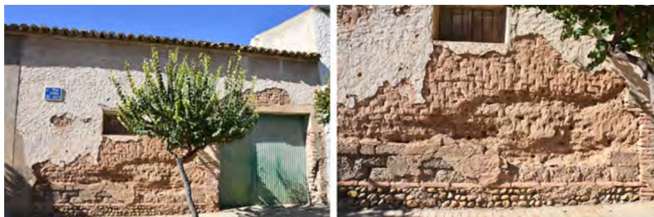
Figure 10. Adobe basement erosion. (Torres de Berellen).
