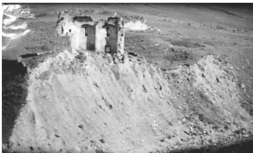
Figure 3. On the photo of 1967 we see only south-eastern half of the building, standing on the edge of the landslide. Photo made by architect V. Kulakov.
