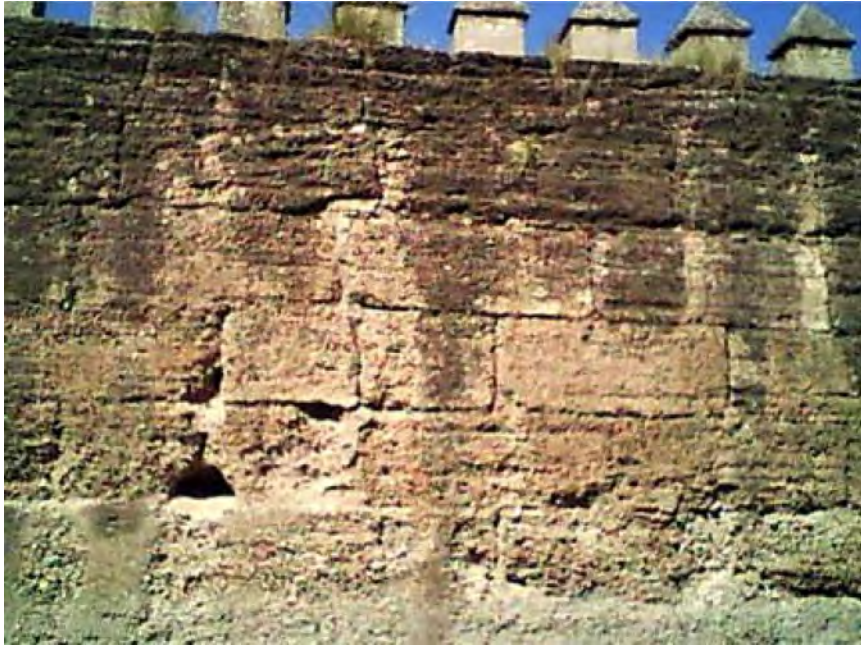
Figure 1. Biological degradation in the Macarena wall.
