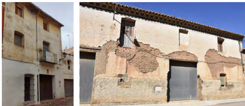
Figure 5. Rammed earth building in Alzira (left). Adobe building in Torres de Berellen (right).
