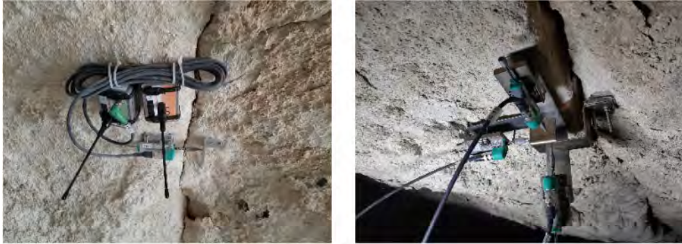
Figure 10. (a) 1D fissurometer (left) and (b) 3D fissurometer (right).
