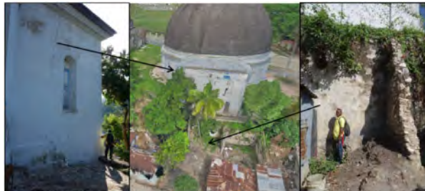
Figure 7. crack in the annex of the chapel (left), 3D view of the Chapel (center, source Iconem) and retaining wall in masonry (right).
