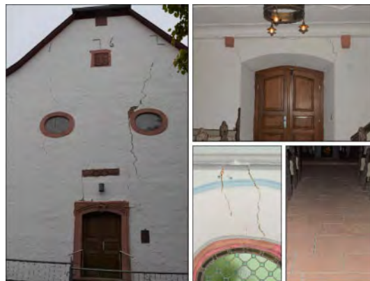
Figure 3. Cracks on the exterior and interior of the west facade and in the floor.
