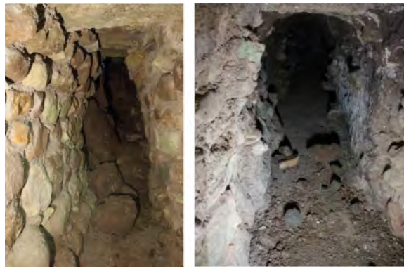
Figure 17. Examples of local collapses: (left) at the interface between lined and unlined stretches; (right) in an unlined tunnel excavated in fine yellow sand ( girín ) (modified after Lacombe et al. , 2020).
