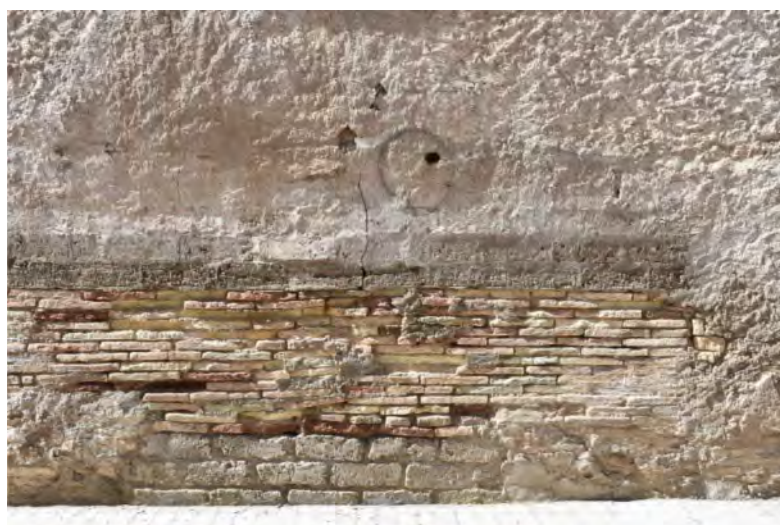
Figure 6. Repair with bricks and concrete blocks in a plinth (Torres de Berellen)
