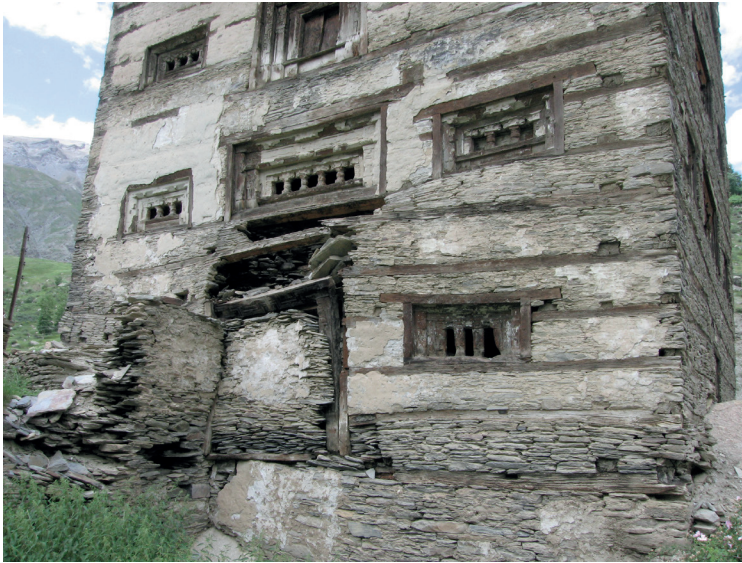
Fig. 4.21 Gondhla. Lahaul. Placing wooden window frames in a stone construction with 'ladder'-like timber lacing.
