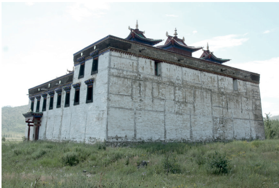
Fig. 4.9 Baldan Bereeven Khiid. Mongolia. Vertical and horizontal timber lacing in a solid wall.
