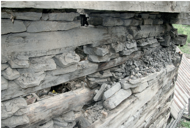
Fig. 4.89 Kalpa. Interior of the kath-kuni wall between the runner beams is filled with rubble stone.
