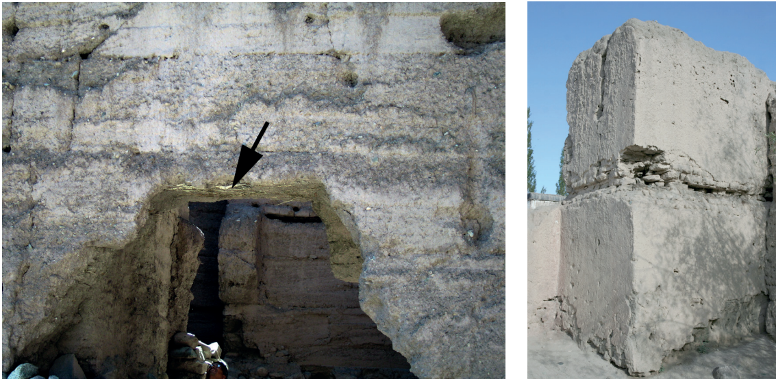
Fig. 4.30 (Left) Saspol. Ladakh. Rammed earth lintel of an entrance gate of the fortress reinforced with twigs.
