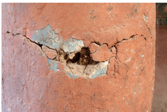
Fig. 3.5 (Left) Basgo, Maitreya Lhakhang. Fibres visible due to a damage of the plaster.
