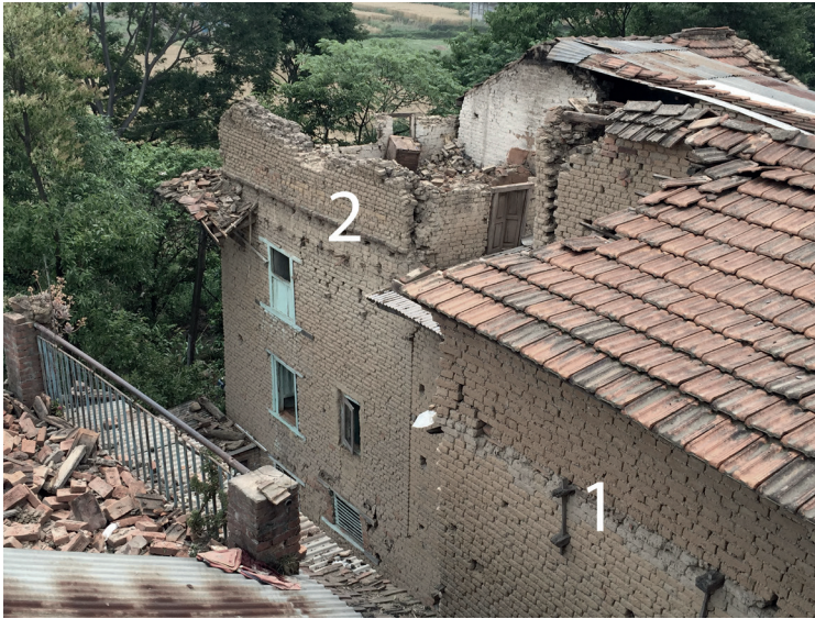
Fig. 4.15 Kathmandu Valley, Nepal. 1 = Wooden wedges as a traditional technique to stabilise walls. 2 = Wooden components destroyed during the earthquake in 2015. Photo: Christof Ziegert.
