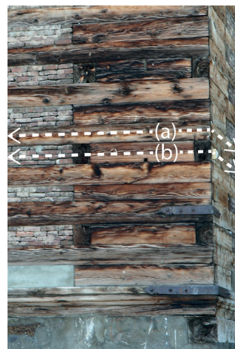
Fig. 4.59 (Bottom) Srinagar. Khanqah-i-Naqshbandi. Corner construction: Runner beams (a) and layers of brick infill (b) are layerwise alternately kept on the same level around the whole building.
