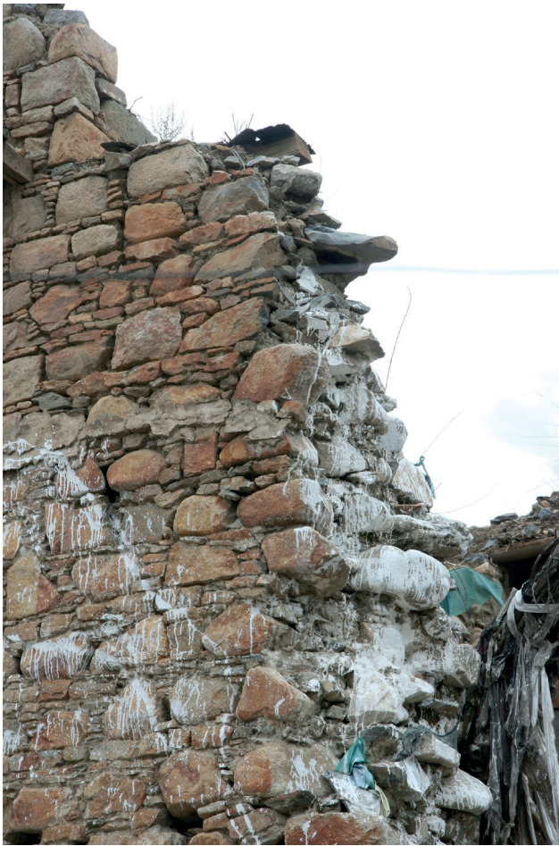
Fig. 4.14 Lhasa, Tibet. Traditional technique of stone laying shown at the Shide Lhakhang.
