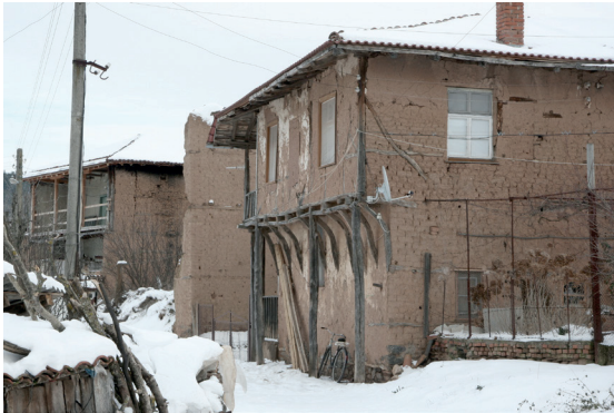
Fig. 4.16 Mandriza. Bulgaria. Adobe brick walls with timber lacing and a projecting upper floor.
