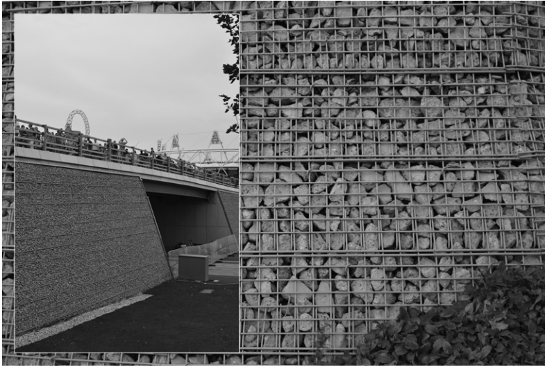
Figure 7.7 Crushed concrete fragments in the facings of the Olympic Park's new bridges.
