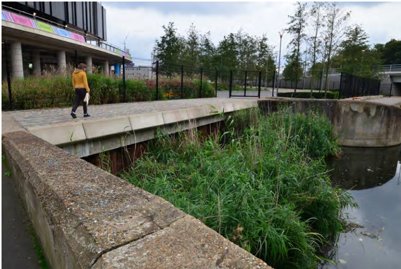
Figure 7.6 The dammed opening of the in-filled Pudding Mill River at its junction with the River Lea.
