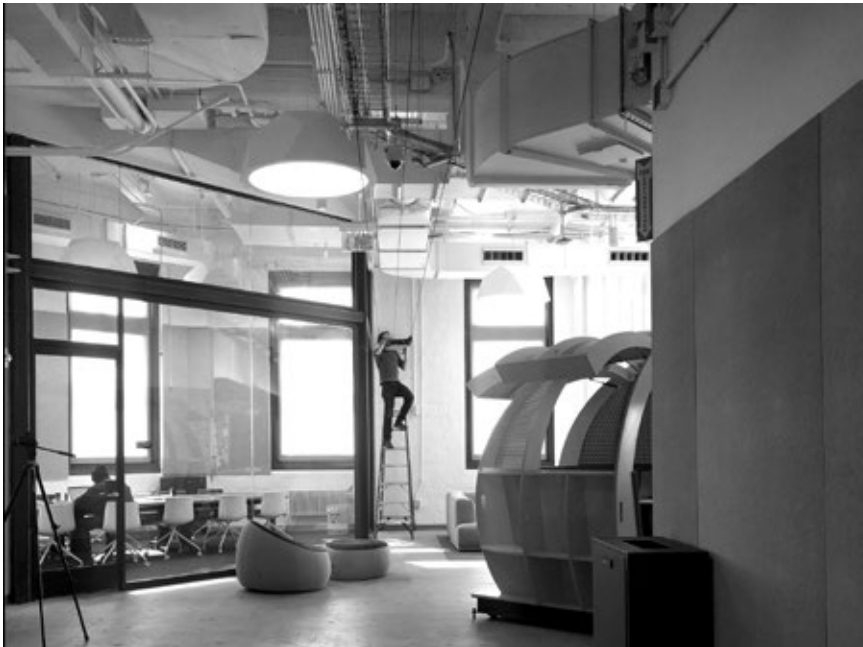
Fig. 3.4 Installation of the railing for the time-lapse in the creative agency’s workspace. Photograph: Pauline Lefebvre.
