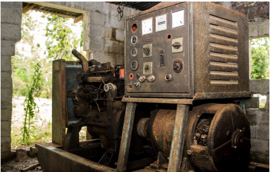
Photo 3. Abandoned electricity generator.
