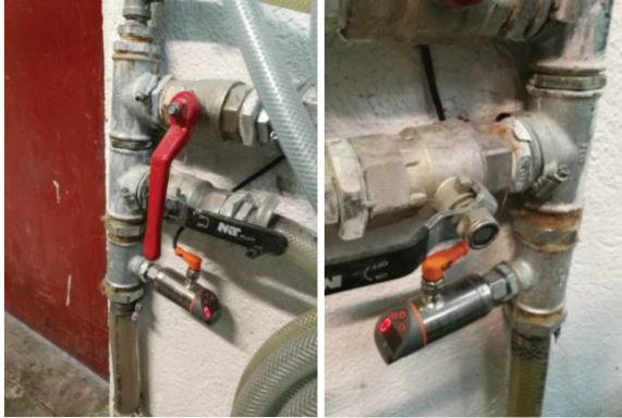
Figure 7.25 Sensors installed in the refrigeration circuit.
