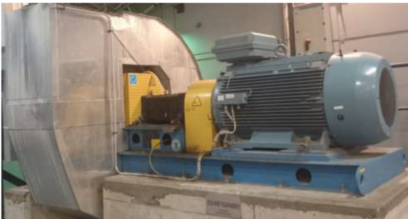
Figure 7.114 Flue gas recirculation blower monitored in the pilot project.
