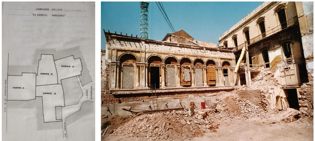
Fig. 08. Identification of the areas subject to restoration and renovation projects (left) and excavation work to create the auditorium level at the street entrance (right) (Project Archive, Matteo Arena Fund, University of Catania, SDS Architecture, Syracuse).
